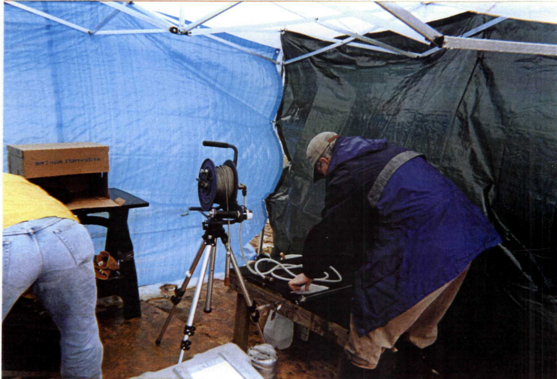
Description: PSARA Technologies, Inc. (PSARA), inside protective tent around monitoring well MW-16
