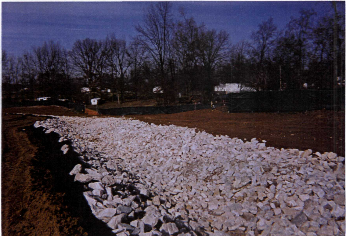
Photograph No. 6 Orientation: Northwest Description: Completed site perimeter drainage ditch on north side of site
