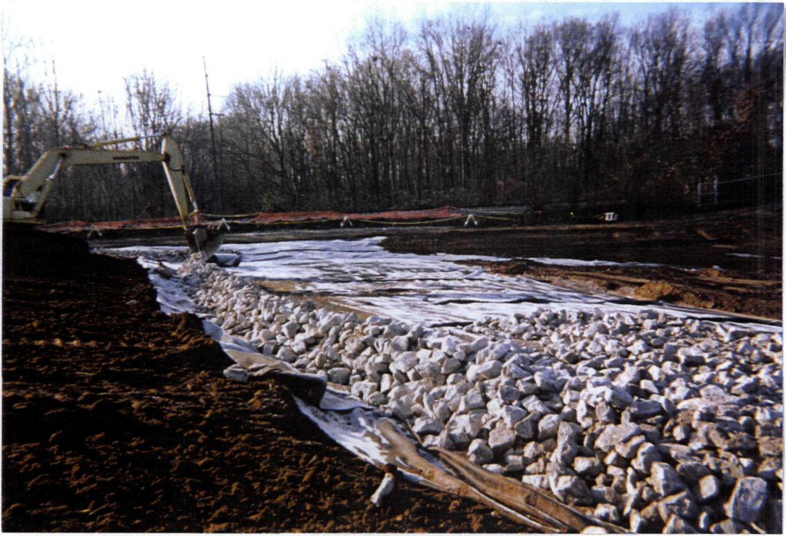
Photograph No. 5 Orientation: South Description: WRS placing riprap in site perimeter drainage ditch
