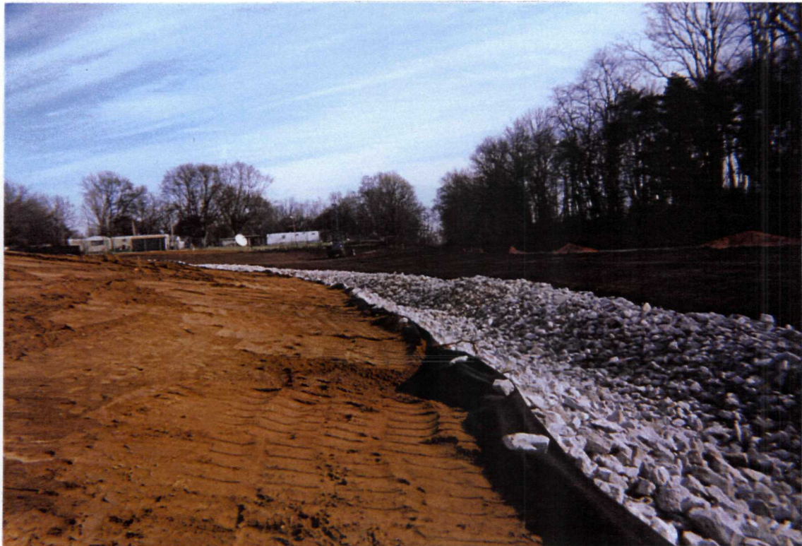
Photograph No. 10 Orientation: East Description: Site perimeter drainage ditch on southeast side, with drilling rig in background
