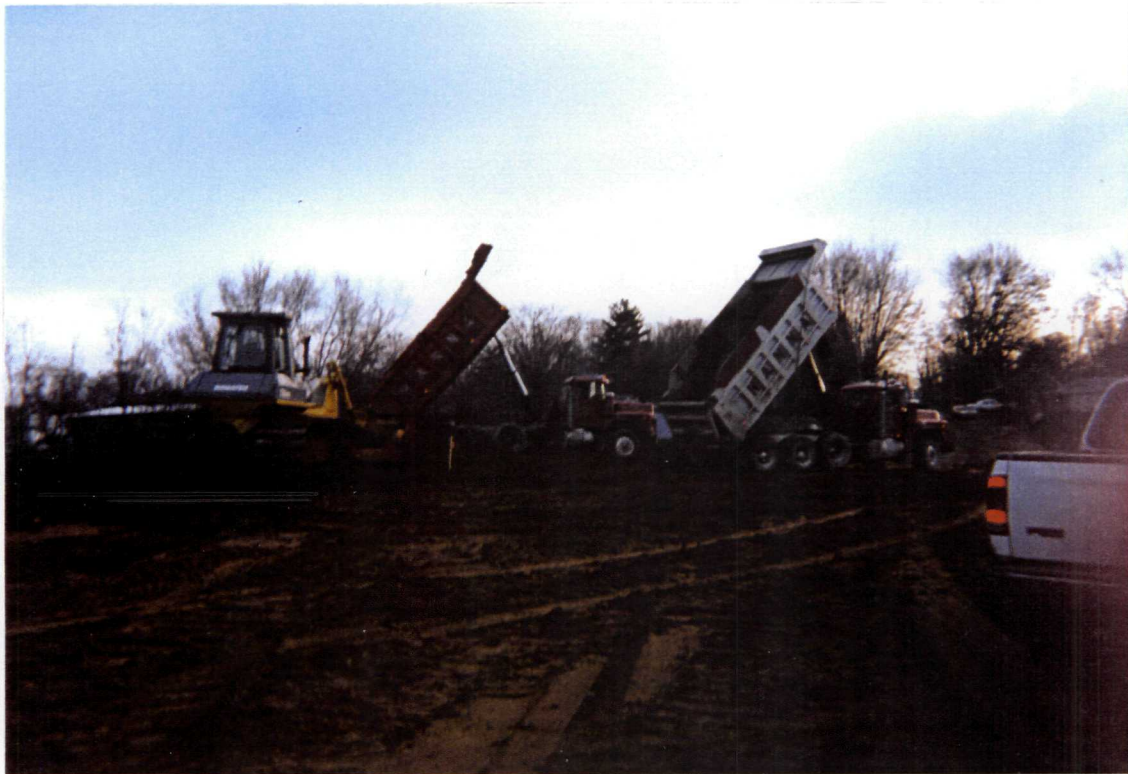
Photograph No. 20 Orientation: Northeast Description: Topsoil delivery to northeast side of landfill cap
