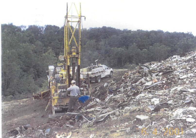
Photo 1. Abandonment of Monitor Well GW-21 near top of landfill.
