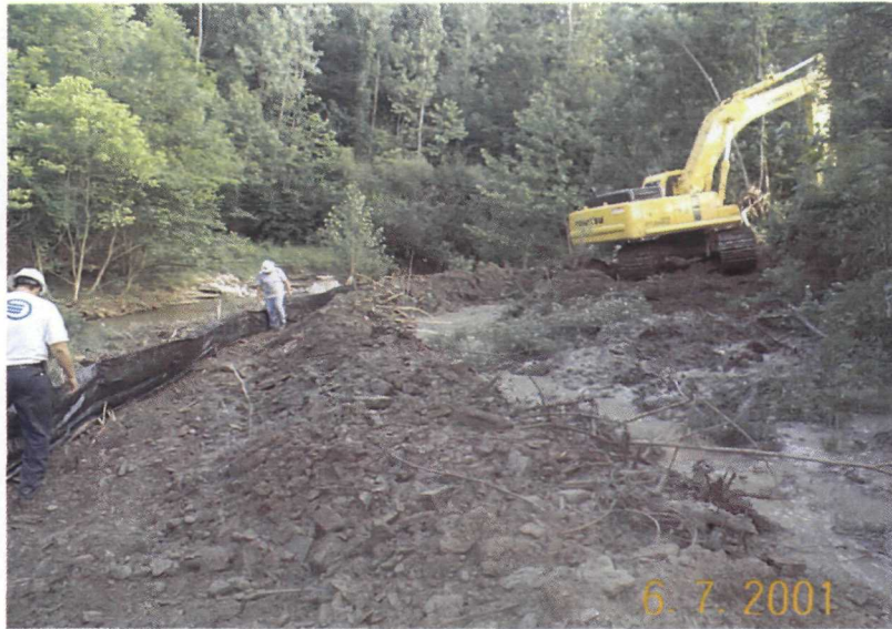
Photo 2 Slurry containment area is shown at right foreground. Silt fence is also shown at left. Butler County Manhole #11 shown in left background.
