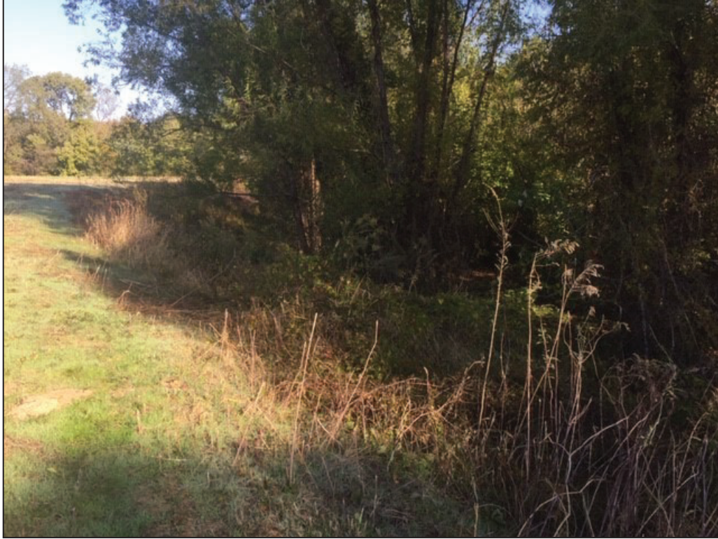
Slope of the East Sector vegetated cap leading to the Wolf River. No visible erosion on slope.
