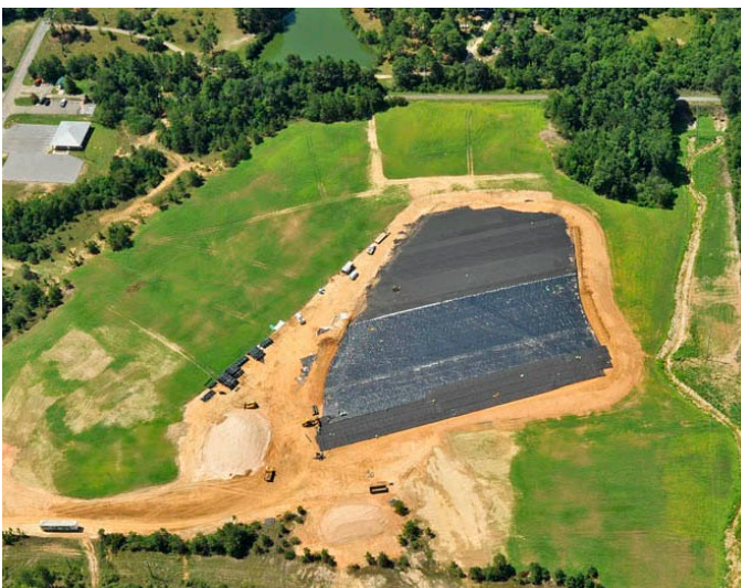
Aerial view of the site during cleanup, 2012. The Longleaf Trace trail is visible at the top of the image, extending from left to right. The black shape is the site's 3-acre impoundment area.
