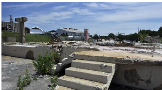
Facility renovations included building demolition. Concrete from this building was reused as road aggregate.
