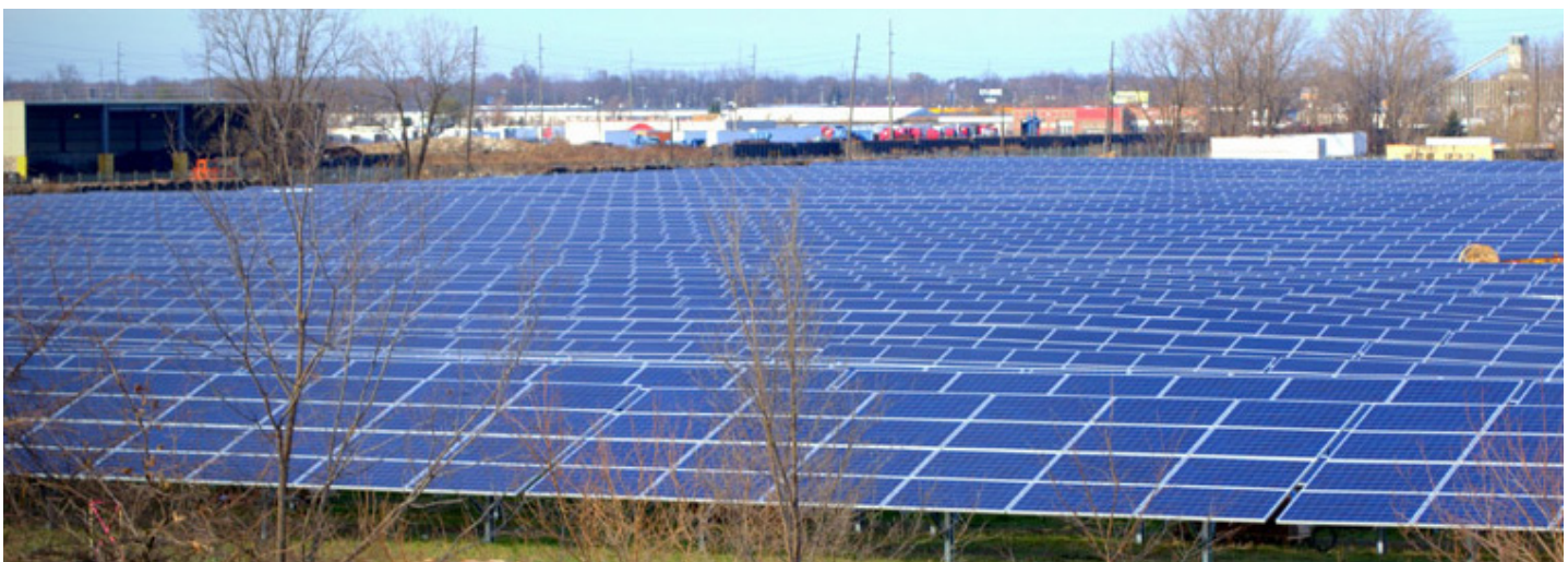
Maywood Solar Farm.
