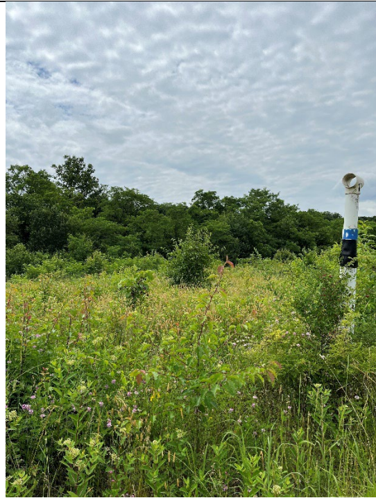
Passive gas vent
