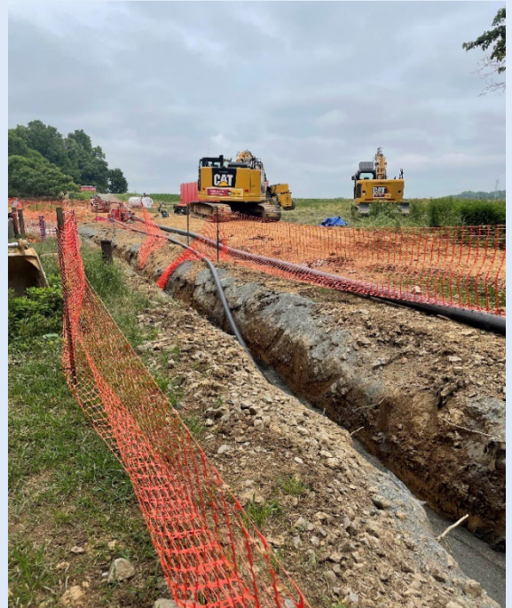
Piping being installed to transport contaminated water from the wells at the source area to the treatment plant.
