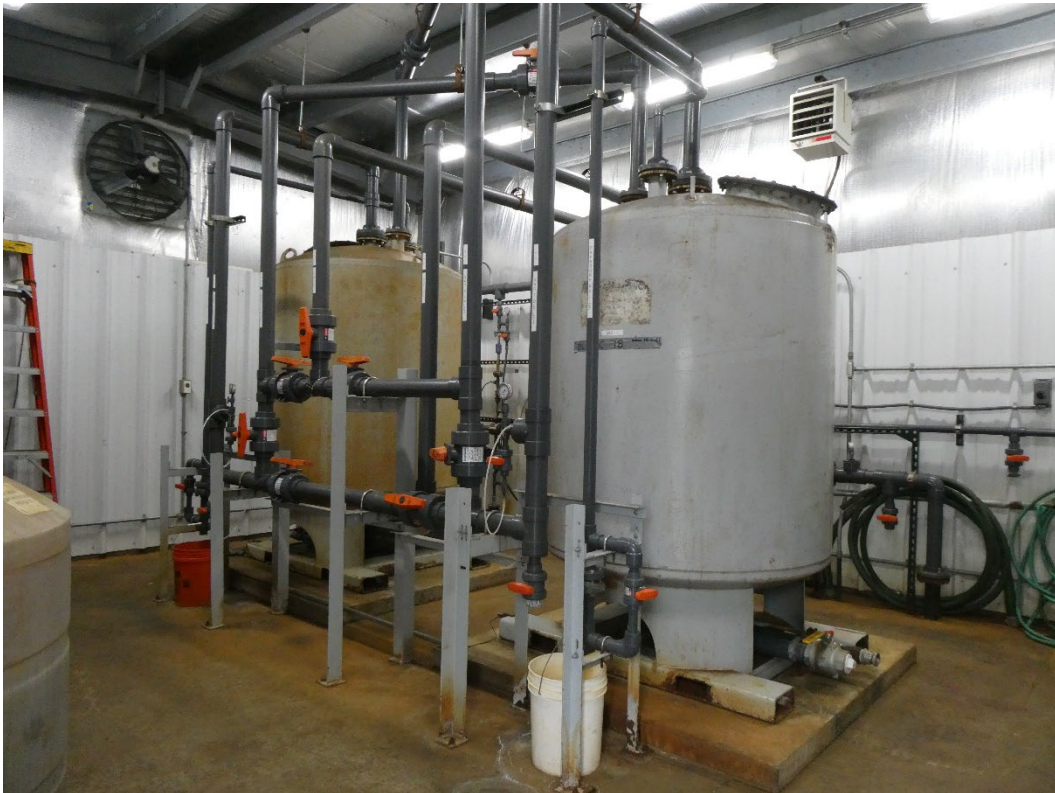
Filters inside the groundwater extraction and treatment building
