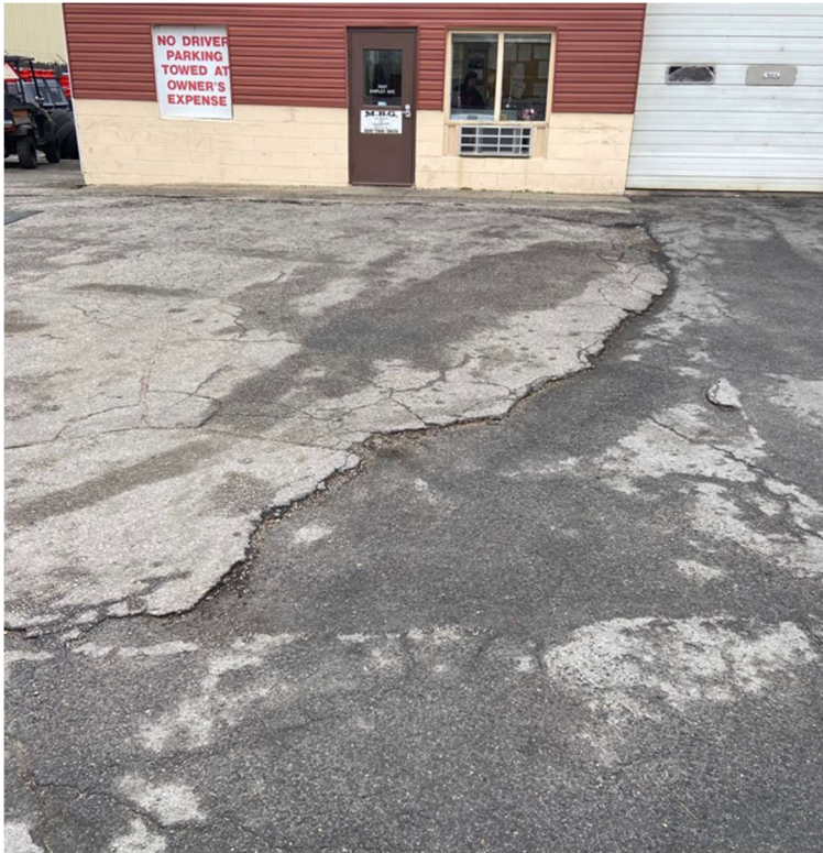
Cracks in the asphalt cap beginning to form around former treatment building – 3/13/2023
