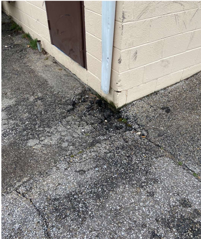
Erosion of the asphalt cap from gutter around former treatment building – 3/13/2023
