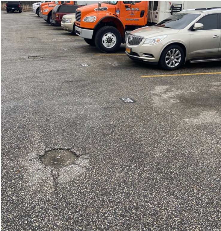
Small holes where propane tank was removed in Treatment Yard – 3/13/2023
