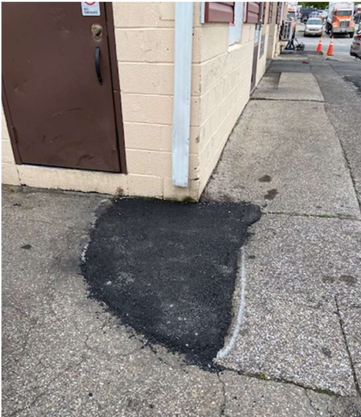
Asphalt repair at gutter around former treatment building - 5/2/2023
