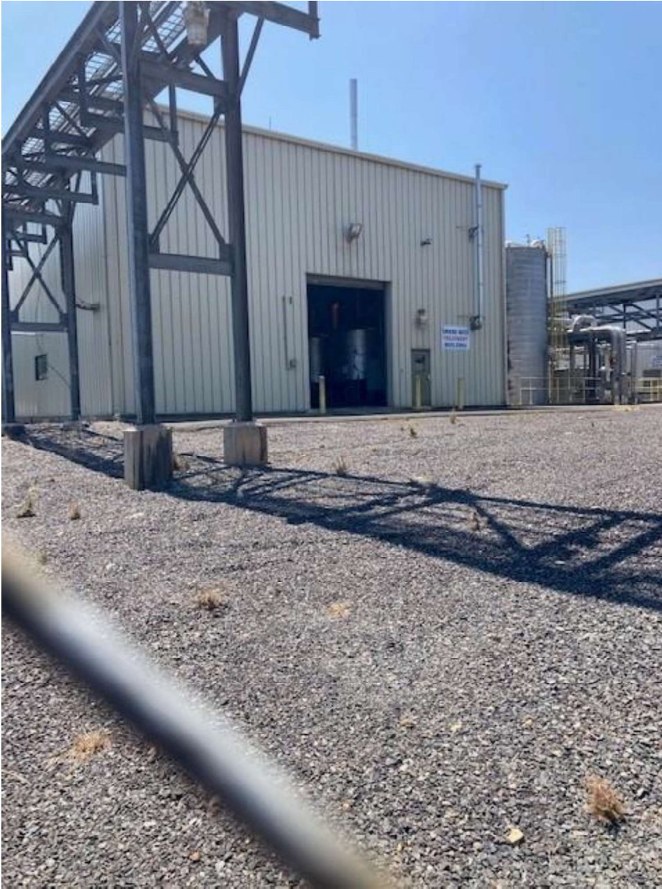
Groundwater Treatment Plant
