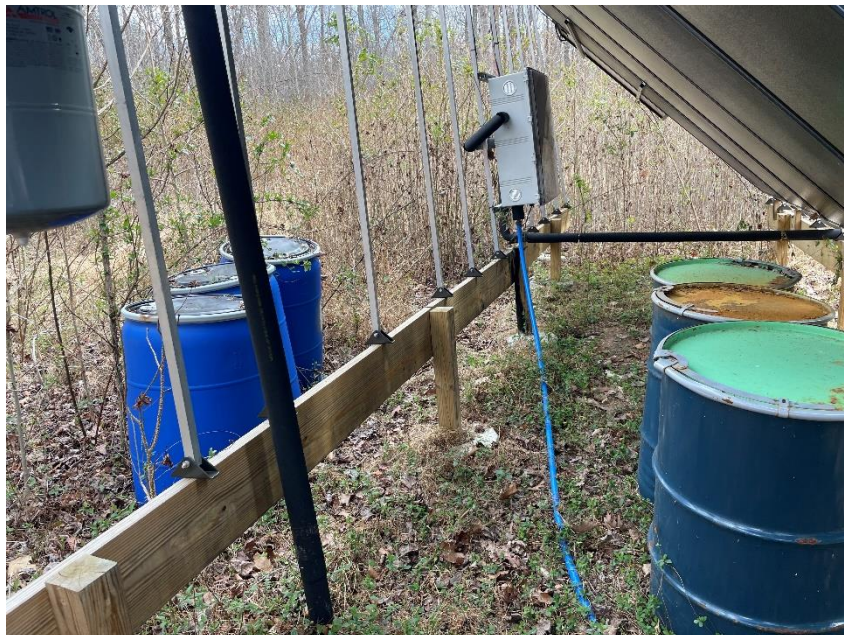
PHOTOGRAPH 06: Empty drums at the solar water heating area. Initial inspection identified the drums as containing some liquid. Subsequent review determined they were empty, but sunk into the ground. Drum to be removed, all liquids handled as per the BARC Master IDW Plan.
