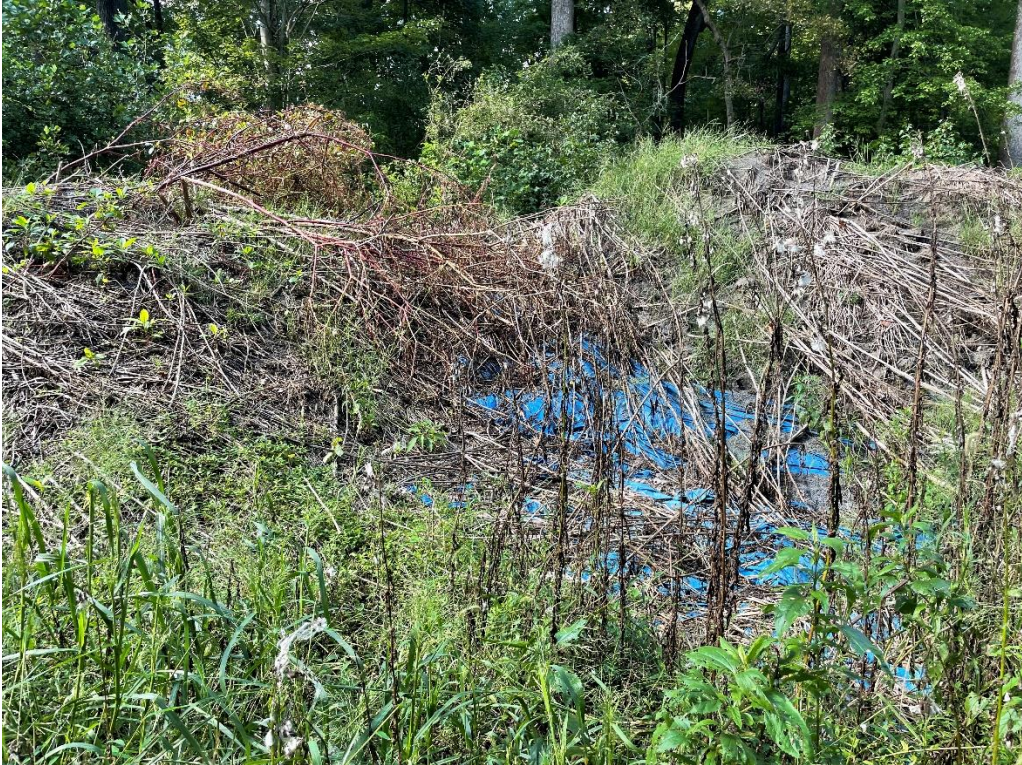
PHOTOGRAPH 06: Excess fill material for upgradient trench pits was stockpiled at the eastern extents of the biowall and covered with a tarp in 2020 to be available for potential system repairs. Tarp should be removed.
