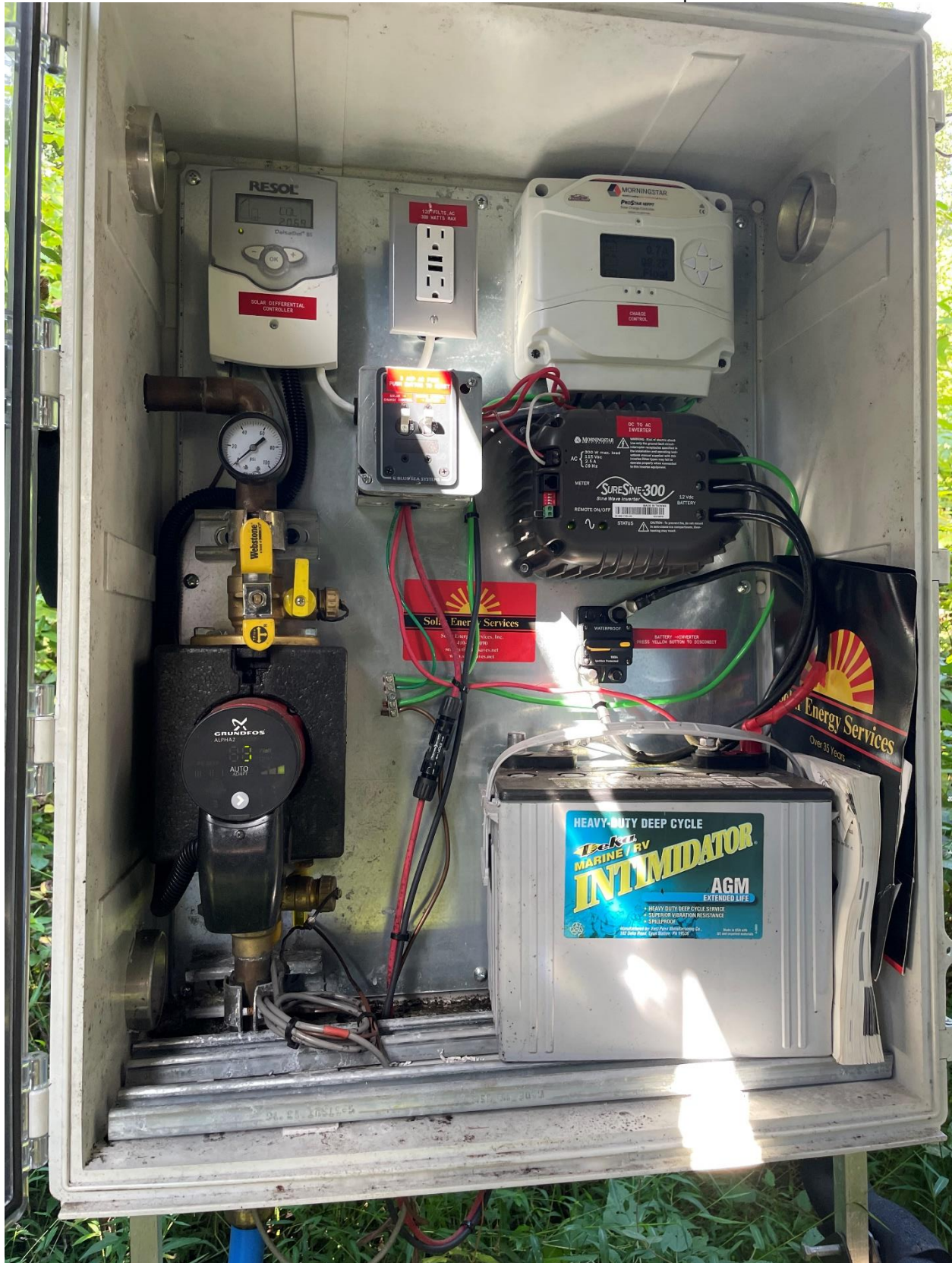
PHOTOGRAPH 05: Solar hot water circulation system main control panel. No signs of tampering or unauthorized access were observed at time of site inspection.
