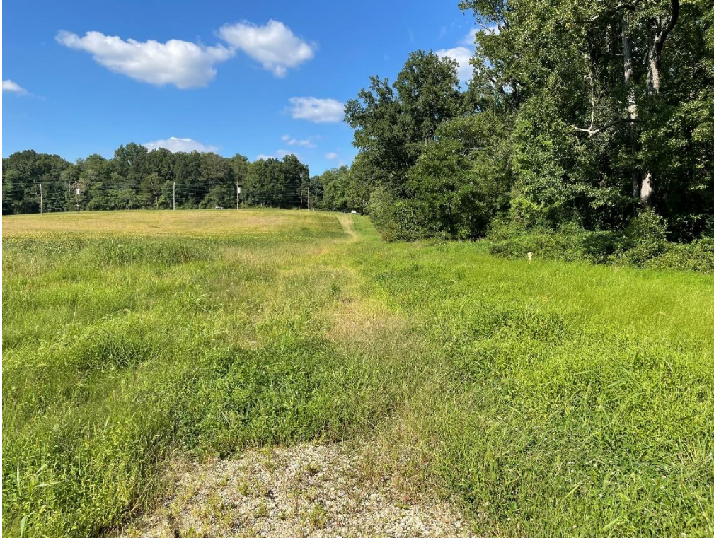
PHOTOGRAPH 08: BDRLF Gravel access road, facing north towards Beaverdam Road from main access gate. Gravel road was in good condition at time of site inspection.
