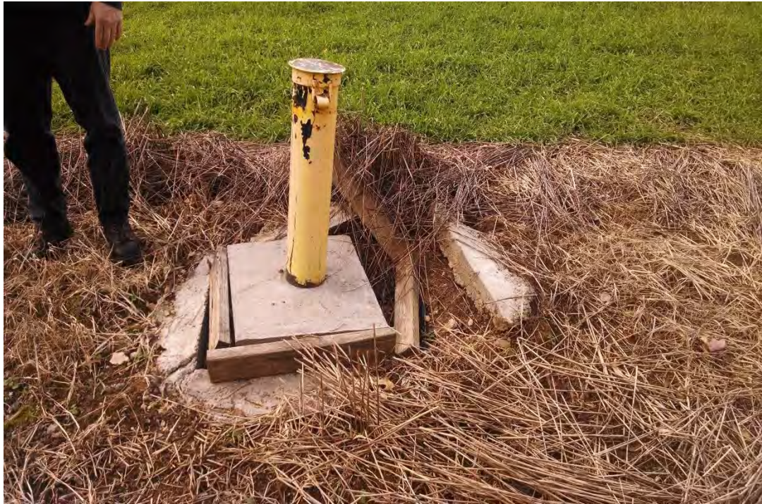
PHOTOGRAPH 04: Damaged Monitoring well MW-4.
