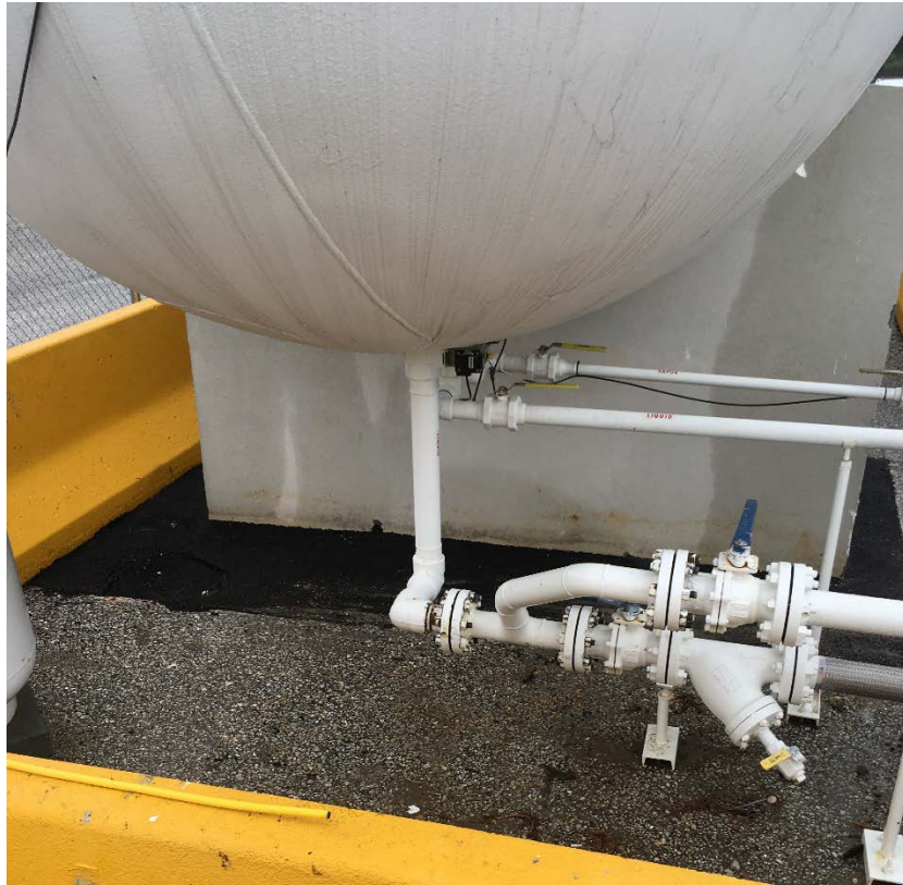
Repaired asphalt from the propane tank installation on the Treatment Year area
