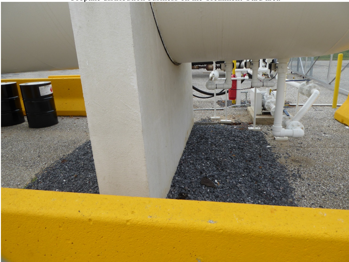
Area where asphalt cap was cut and removed during propane tank installation at the Treatment Yard area
