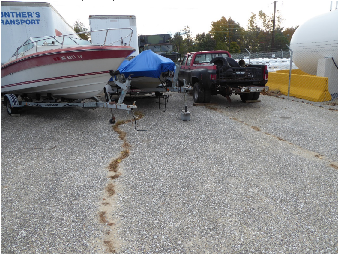
Cracks in the asphalt cap at the Treatment Yard area
