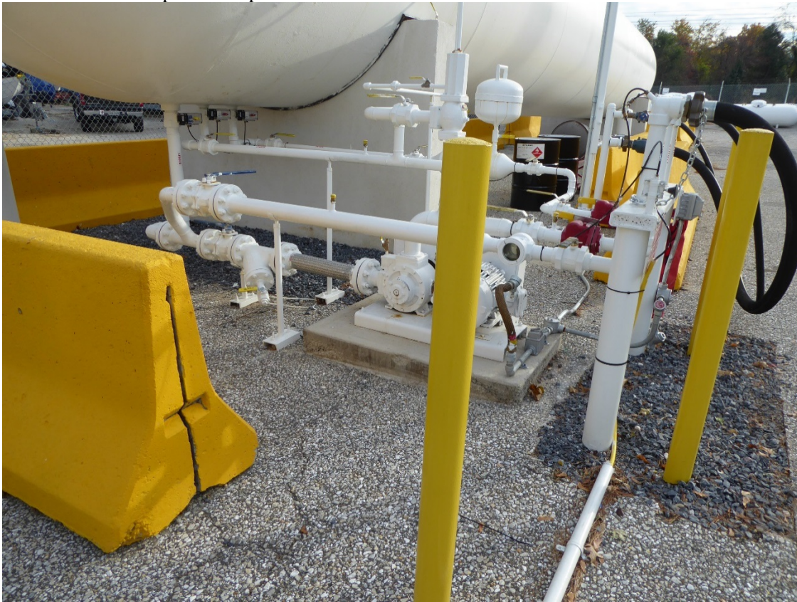
Areas where asphalt cap was cut and removed during propane tank installation at the Treatment Yard area
