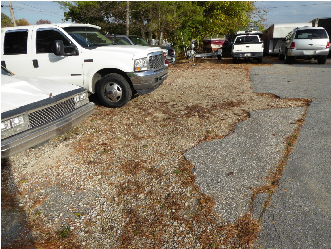
Deteriorated asphalt at the front of the Treatment Yard area
