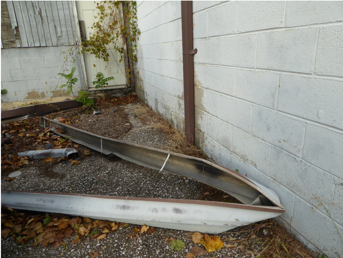
Damaged rain gutter at the Treatment Yard area
