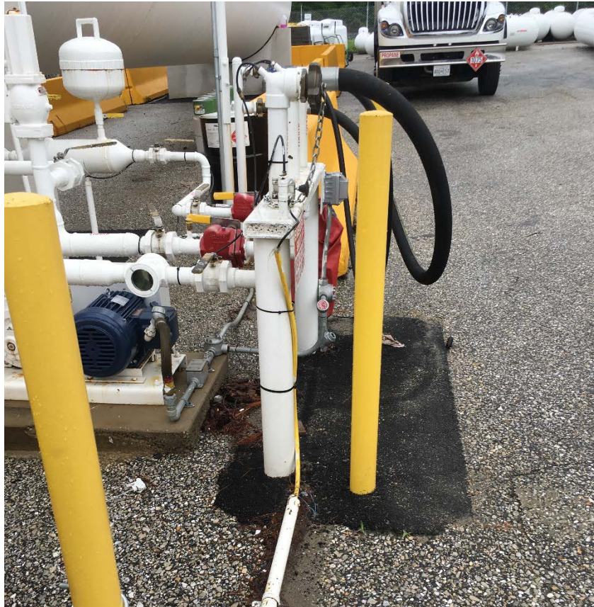
Repaired asphalt from the propane tank installation in the Treatment Yard area
