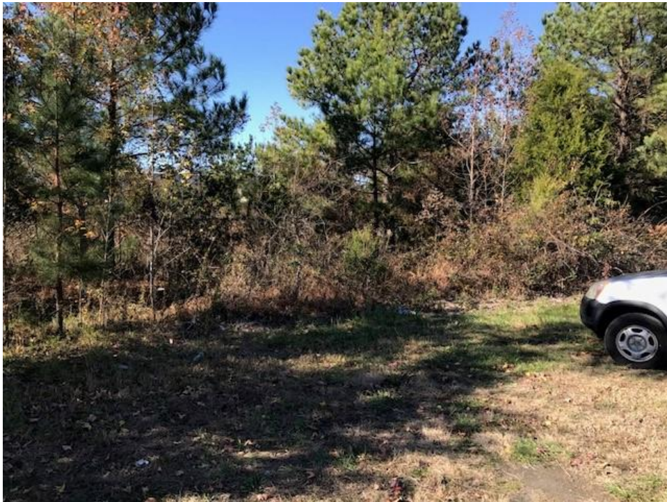
Overgrown drainage ditch area
