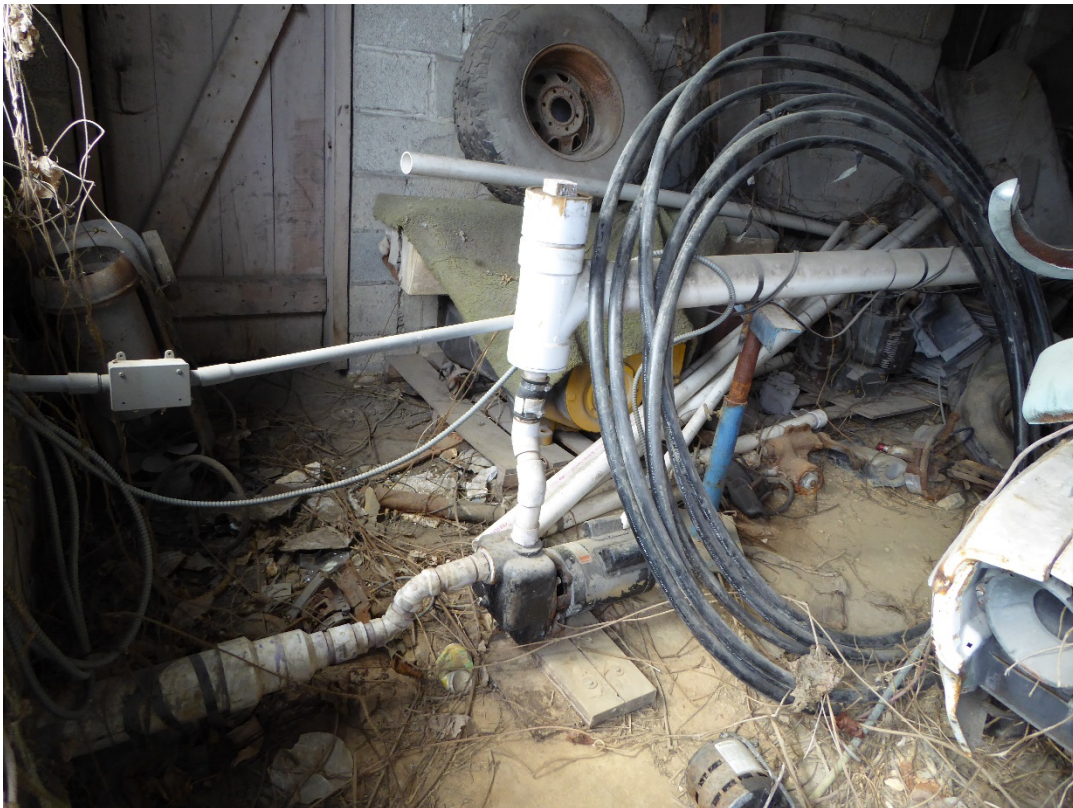
Groundwater extraction components (shut down in April 2017)
