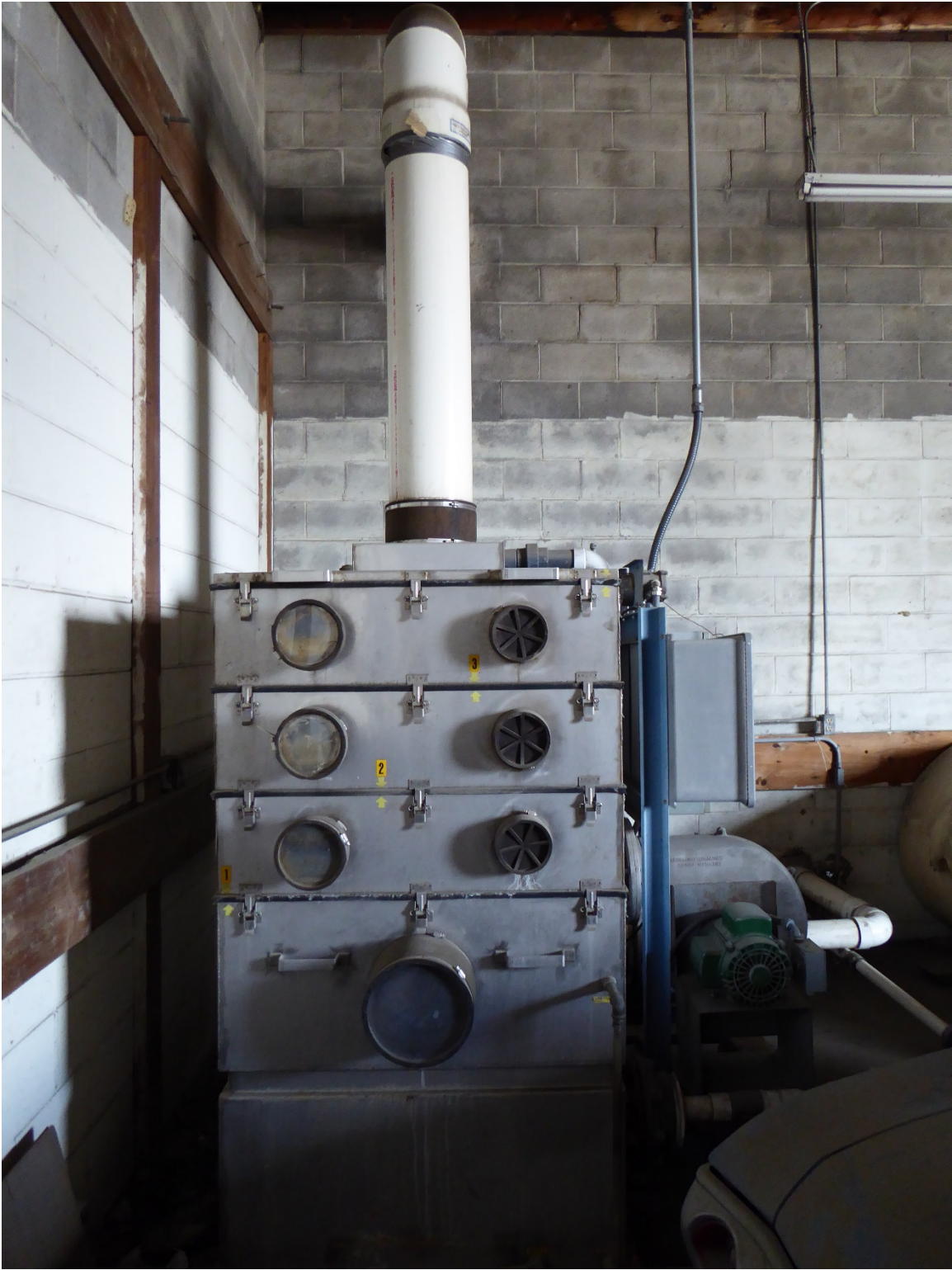
Air stripper (shut down in April 2017)
