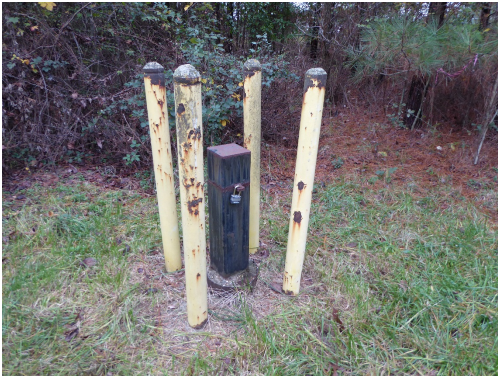
VPMW-4 (not labelled and has cracked concrete base)
