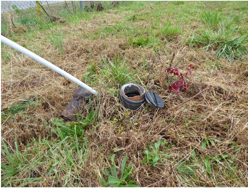
Damaged sanitary sewer tie-in along Peyton Street cap edge
