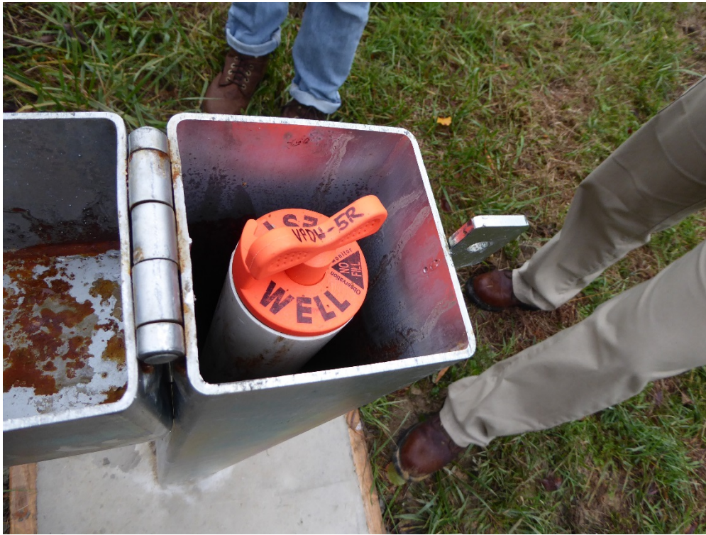
New monitoring well VPDW-5R
