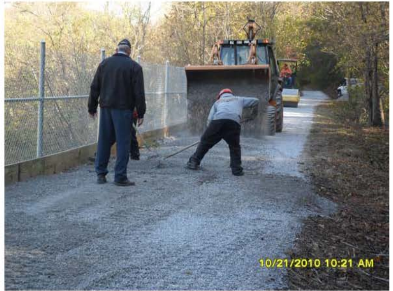
10/21/2010 In preparation for paving, ERRS placing crush-n-run on trail to build a level base. SAM_0026.JPG
