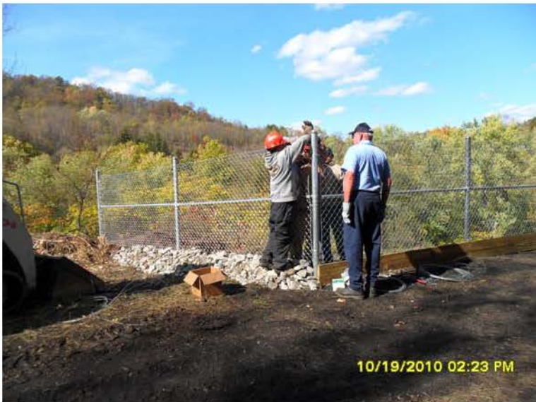
10/19/2010 ERRS installing tension wire on top section of chain link fence. SAM_0011.JPG
