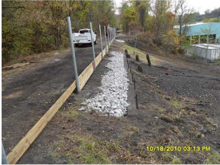
10/18/2010 View of area behind the fence. SAM_0007.JPG
