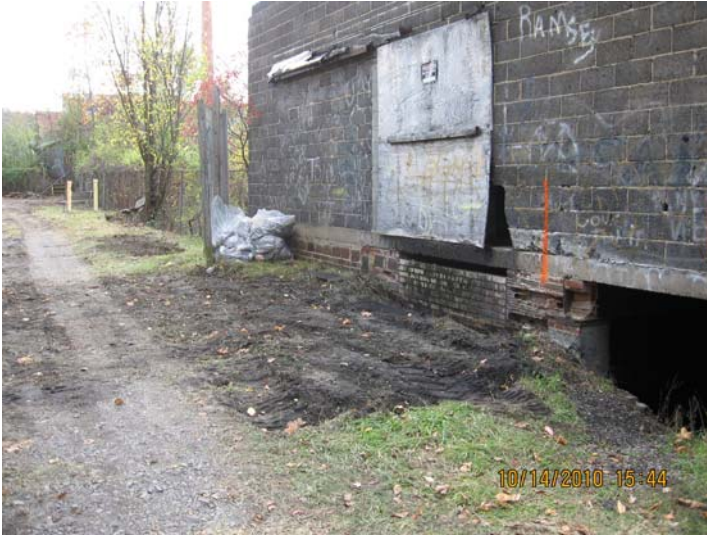
10/14/2010 Area where ERRS removed RR ties from head of trail (SSW) IMG_5493.jpg
