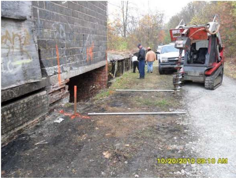
10/20/2010 ERRS preparing for the installation of a fence adjacent to the building SAM_0017.JPG
