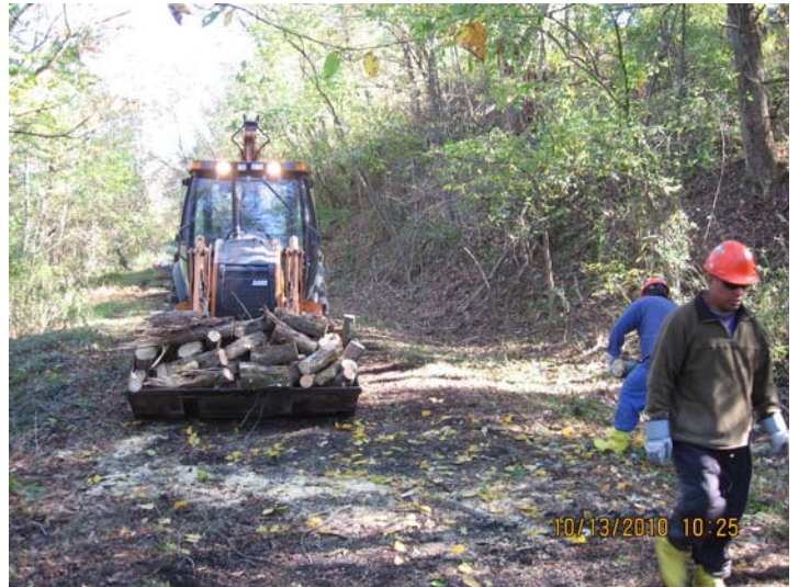
10/13/2010 ERRS using excavator to move cut wood to staging area - (N) IMG_5469.jpg
