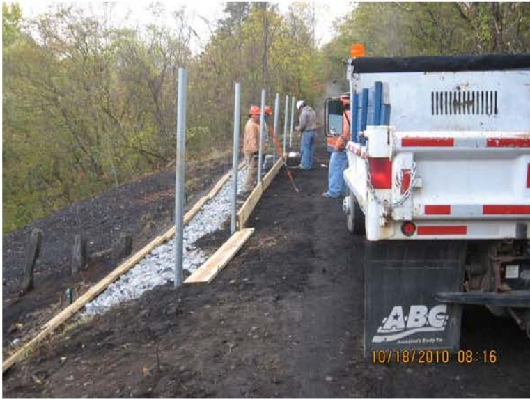
10/18/2010 ERRS installing wooden boards at base of fence. The trail will be covered with aggregate. Uh IMG_5564.JPG
