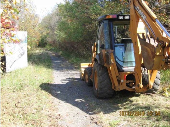
10/12/2010 Rails to Trails trail upon initial ERRS entry and work (North) IMG_5435.jpg
