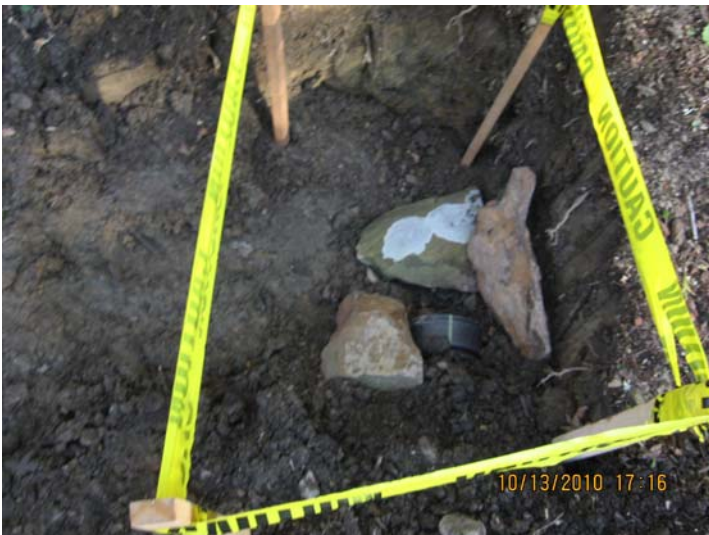
10/13/2010 Head of installed drain pipe - water will cross from (E) to (W) IMG_5482.jpg
