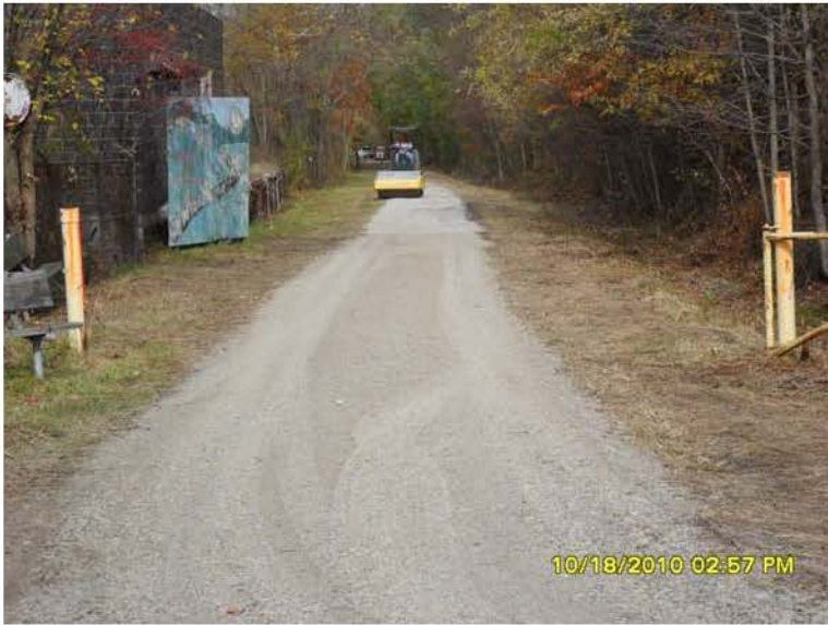
10/18/2010 ERRS rolling/compacting gravel base on trail in preparation of asphalt being Udd`YX SAM_0004.JPG
