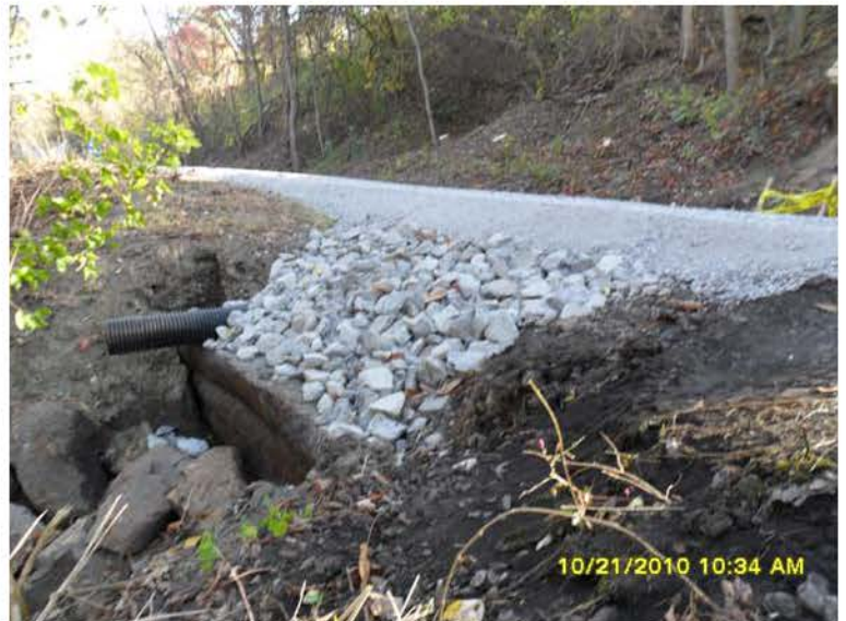
10/21/2010 View of drainage pipe which runs underneath trail. SAM_0028.JPG
