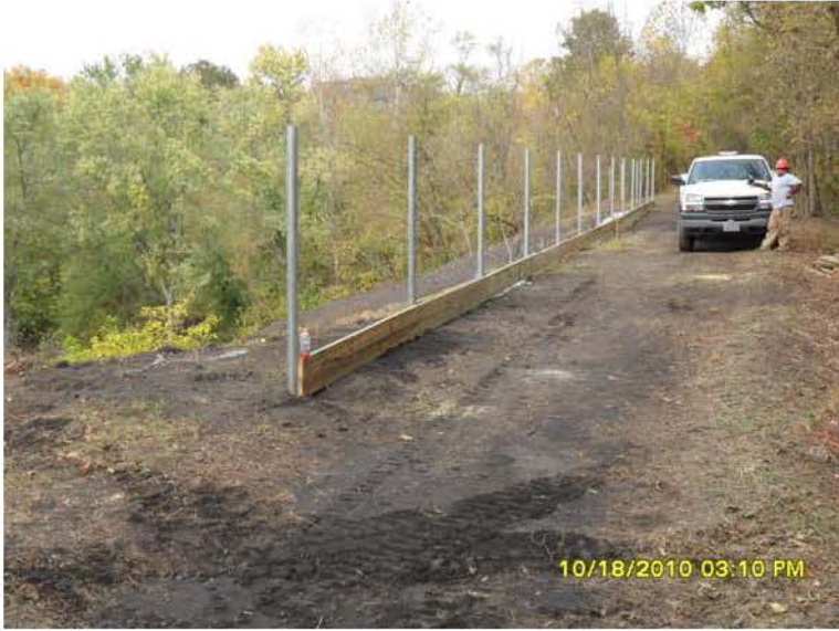
10/18/2010 Progress of the installation of wooden boards at base of the fence. SAM_0006.JPG
