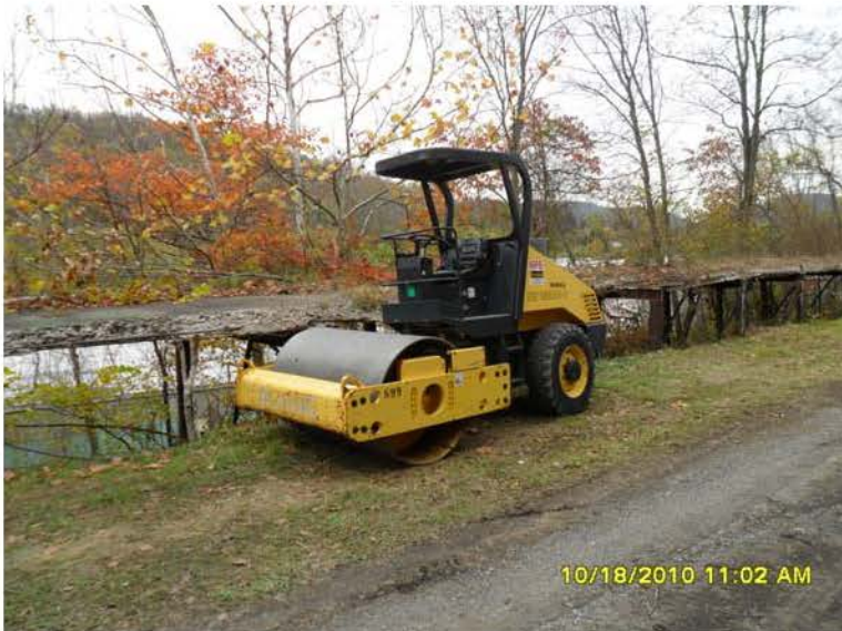
10/18/2010 Photo of compactor/roller which is being used to compact gravel base of trail. SAM_0002.JPG
