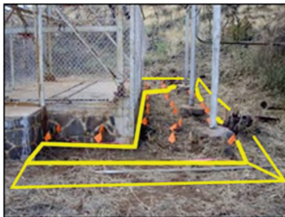
Figure C-1. Decision Unit designated to investigate PCB contamination beside former transformer pad. Boundary DUs to confirm edges of contamination.
