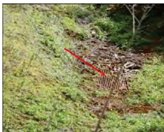
Figure C-14. Stormwater drainage vault designated as a DU for testing of sediment runoff from a contaminated property.
