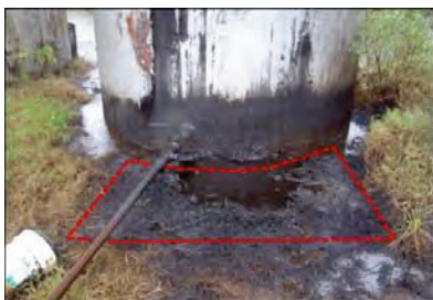
Figure C-13. Stained area under valve of large fuel tank designated as a small DU to document the presence of a release.
