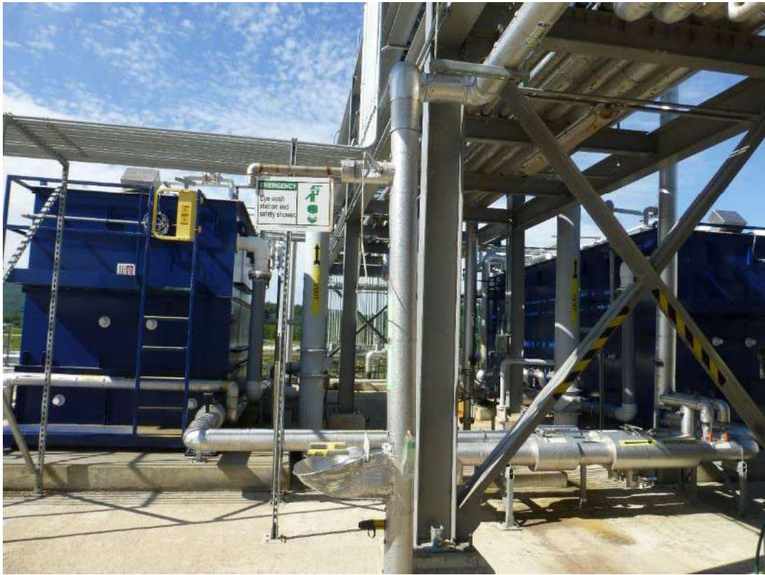
Metals precipitation tanks on the tank deck at the GLTP
