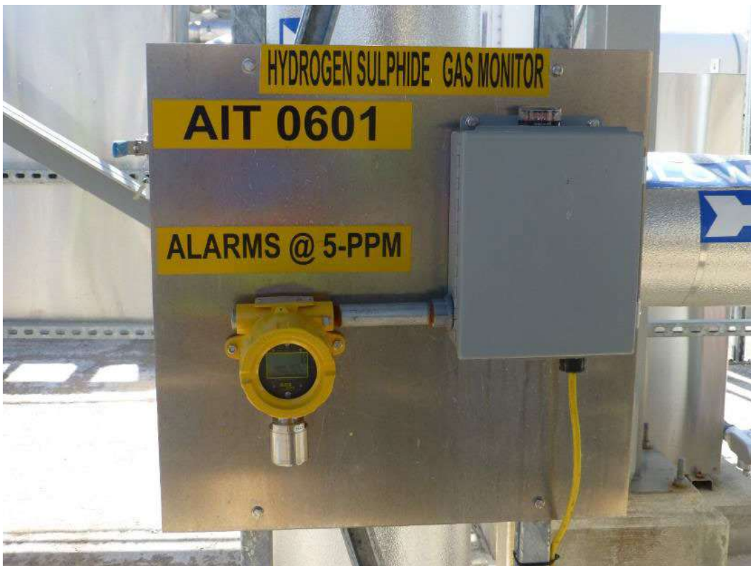
Hydrogen sulphide gas monitor on the tank deck at the GLTP
