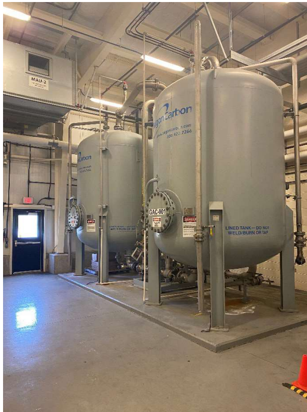
Carbon filtration units inside the GLTP
