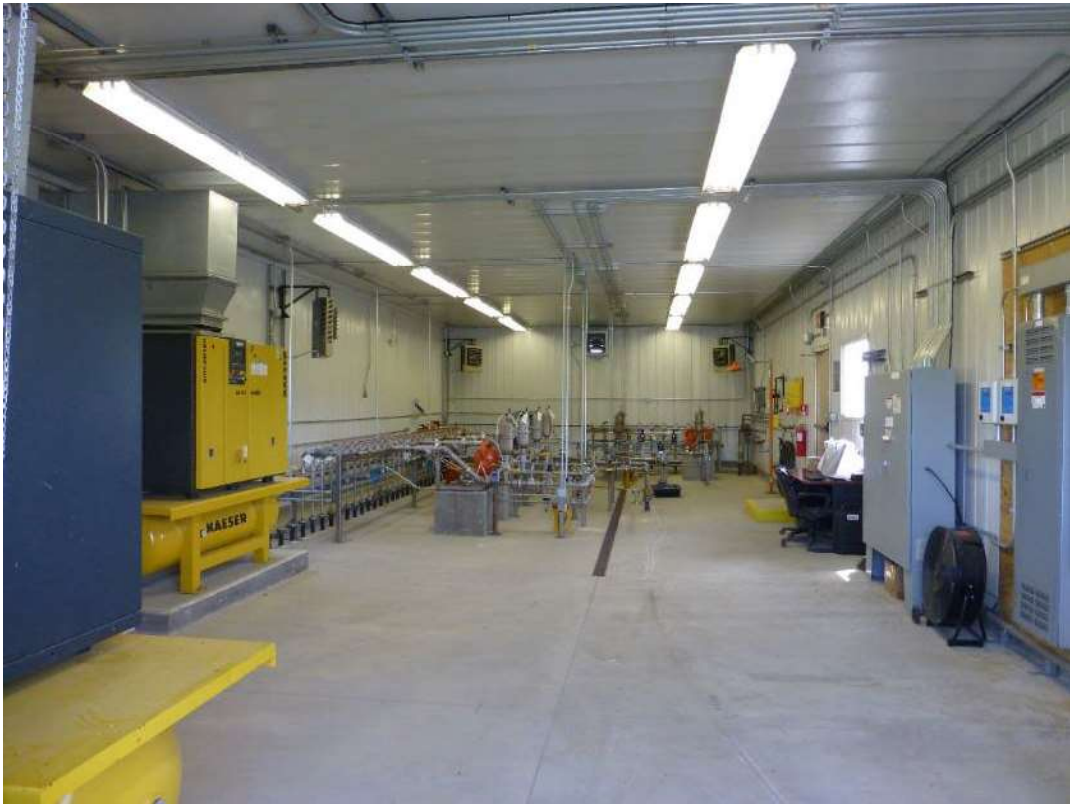
Interior of the VB extraction equipment building
