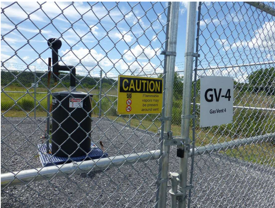
Carbon filtration unit installed on VB 5 at OU10 GV-04
