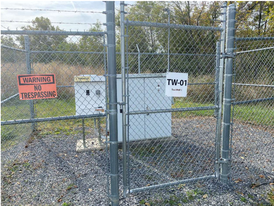
Deep groundwater extraction well TW-01
