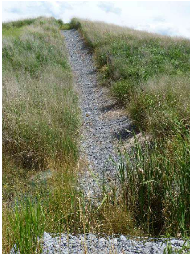
VB 6 stormwater discharge chute
