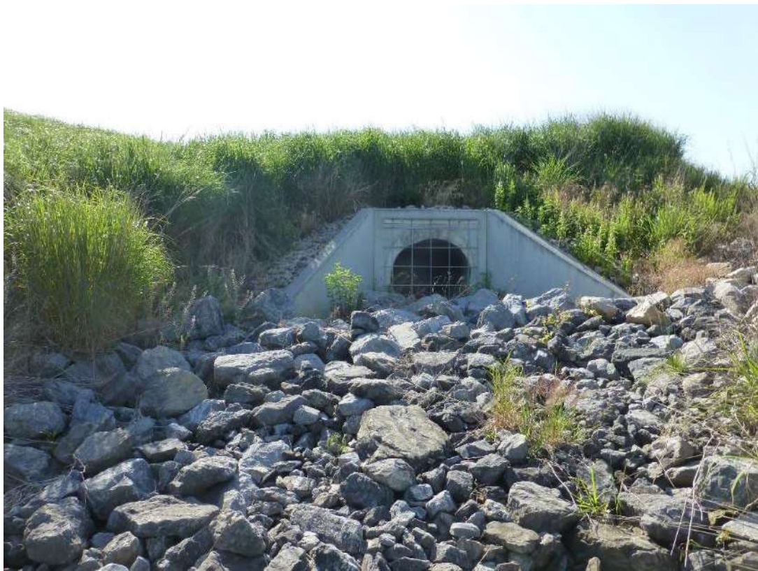
Stormwater discharge outlet at SB 2
