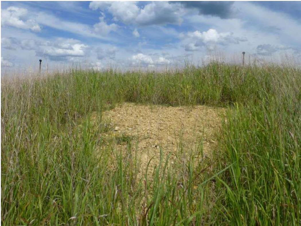
Previously unidentified bare spot observed on SB 3 near GV-8. The PRP is aware of the maintenance issue and plans to address the issue in the fall of 2017
