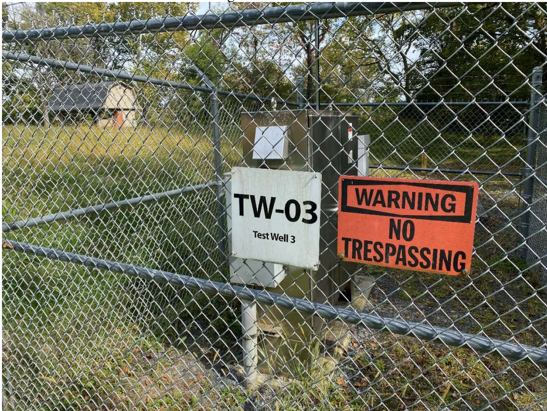
Deep groundwater extraction well TW-03, located within a locked enclosure on the west side of the river
