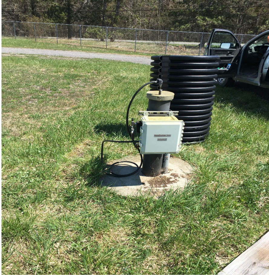
Photo of Remedial Pumping Well – East Side
