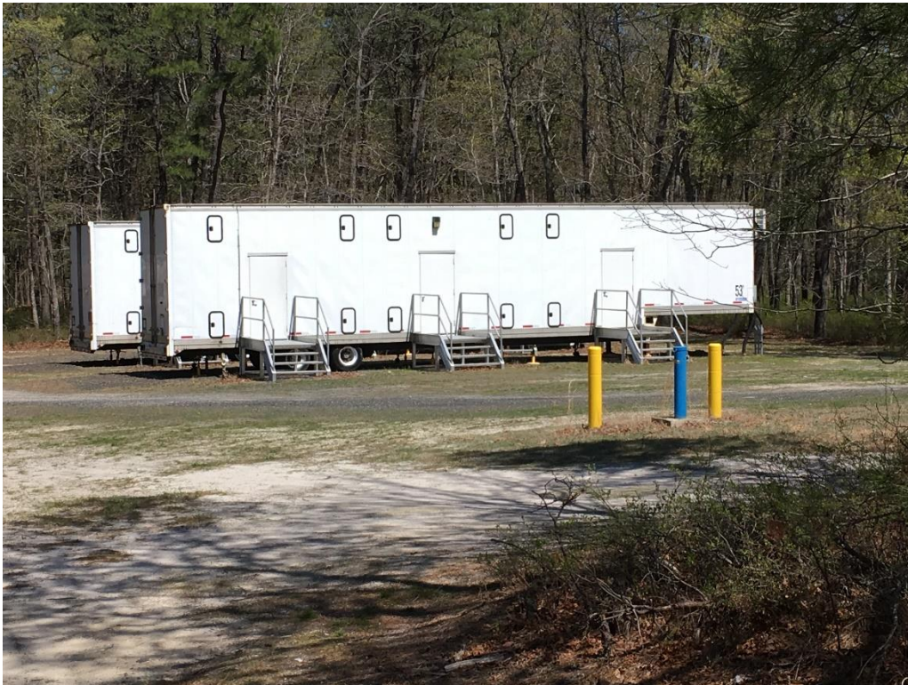
OU02 - Area 20A treatment trailers
