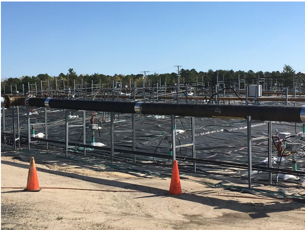
OU01 - Area D, Phase I Thermal Conductive Heating System
