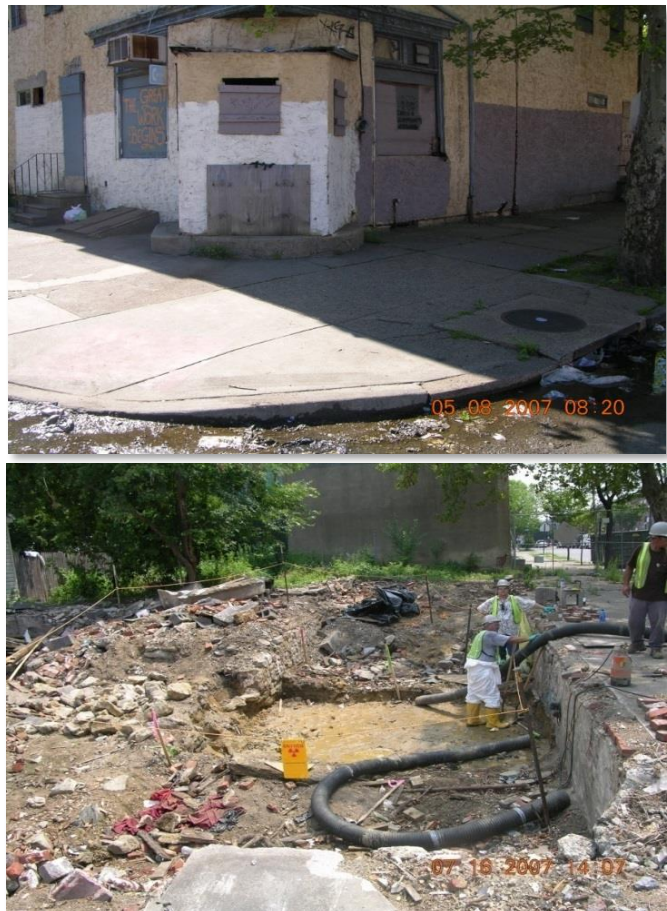
Figure 3. An abandoned pub (top) was demolished and the area excavated (bottom) to prepare the site for reuse as a professional theatre.
