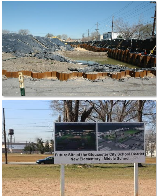
Figure 4. Remediation of a property for a much-needed future elementary and middle school.
