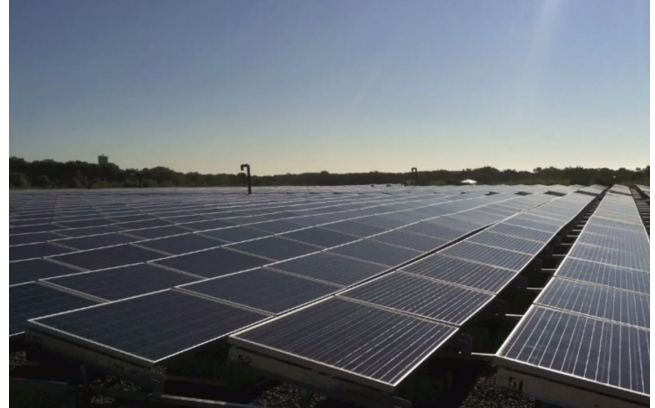
Mounted solar panels on the cap.
