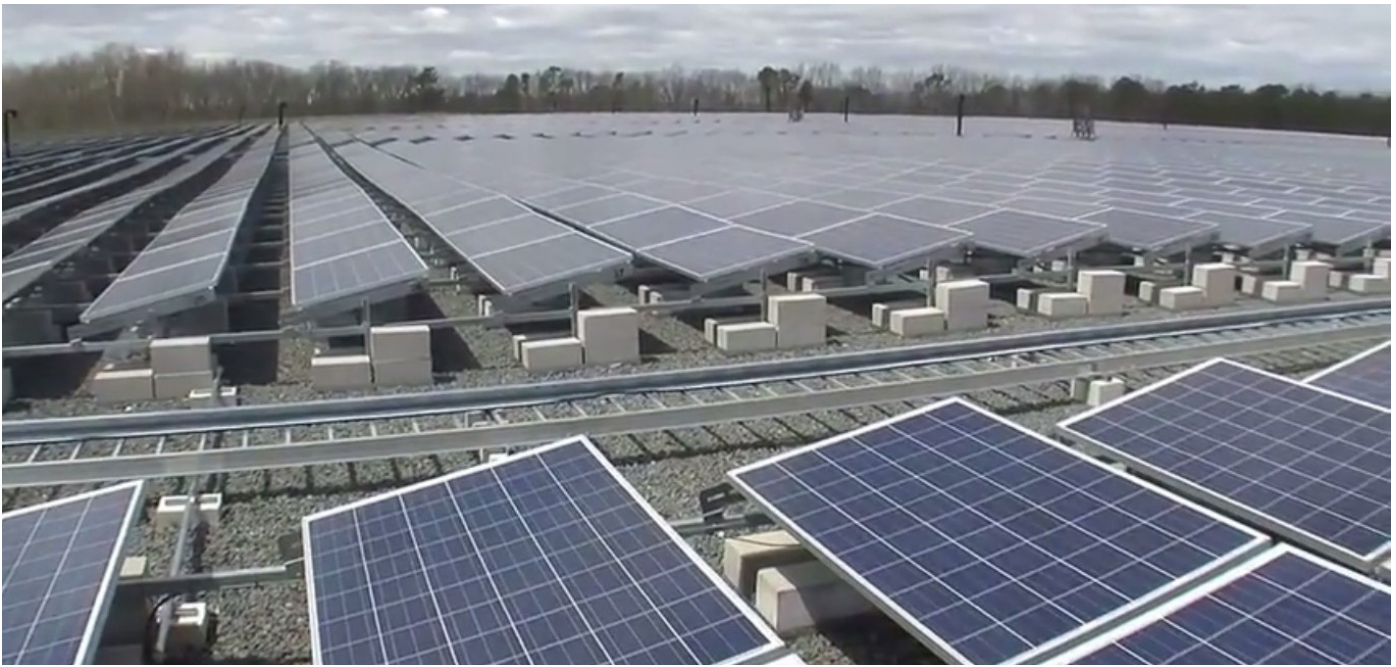
Skid-mounted PV solar panels installed at the site.
