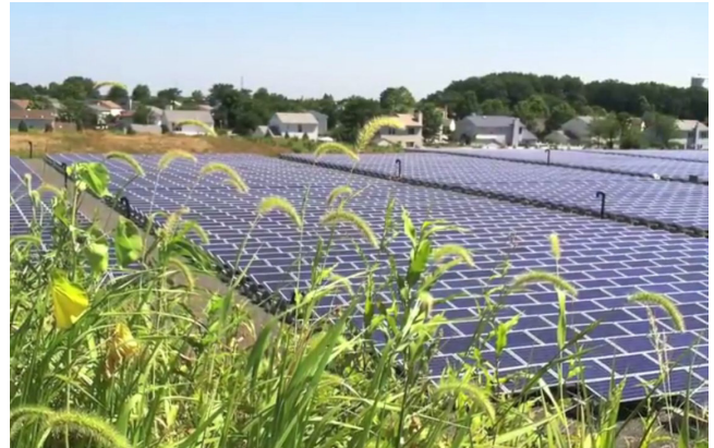
Solar panels at the Brick Township Landfill site.
