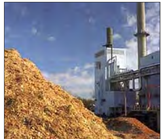
The McNeil biomass-fired power plant, located in Burlington, Vermont's Intervale eco-industrial park, is operated by the city-owned utility Burlington Electric Company.
