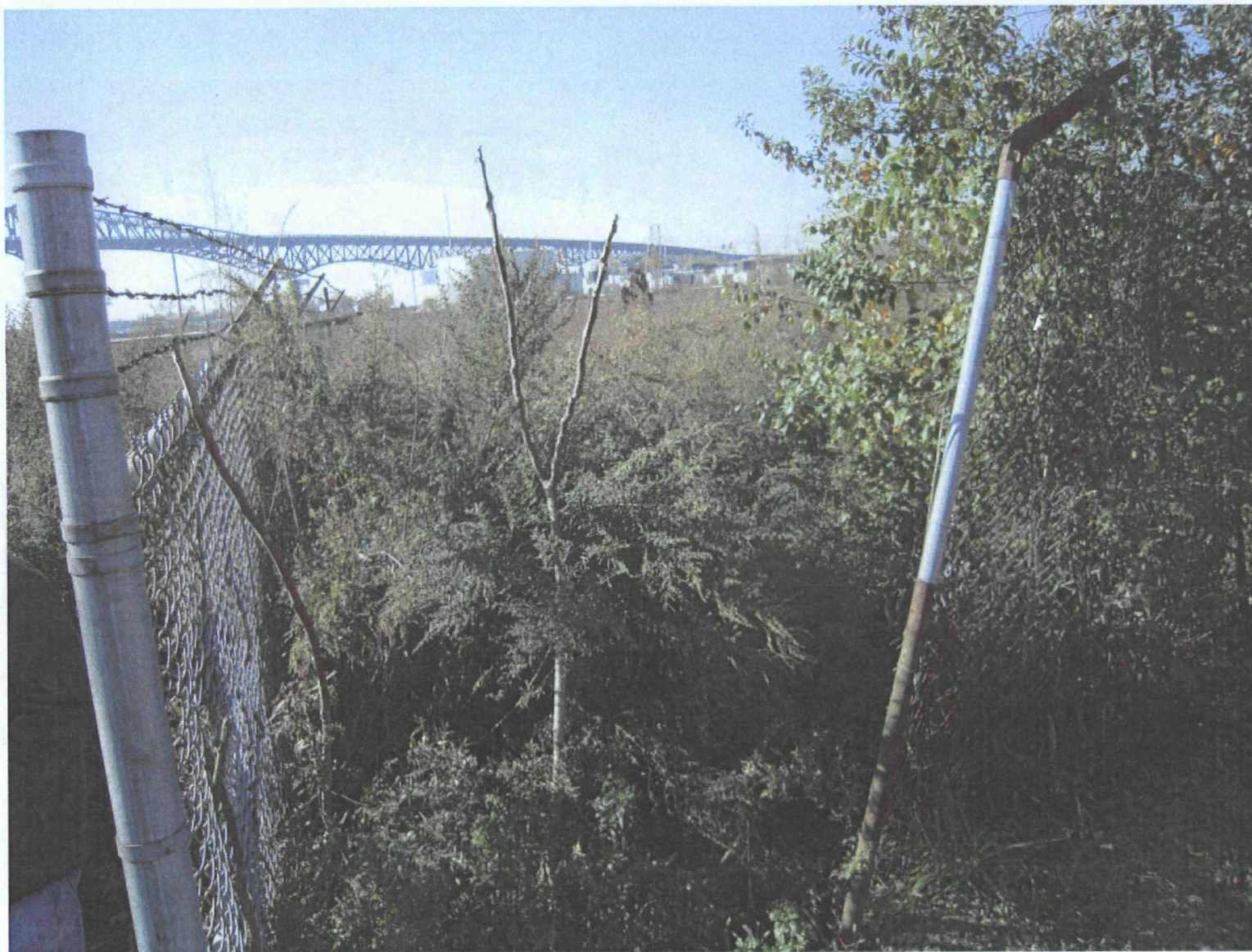
Figure 5 - Gap in Fence
