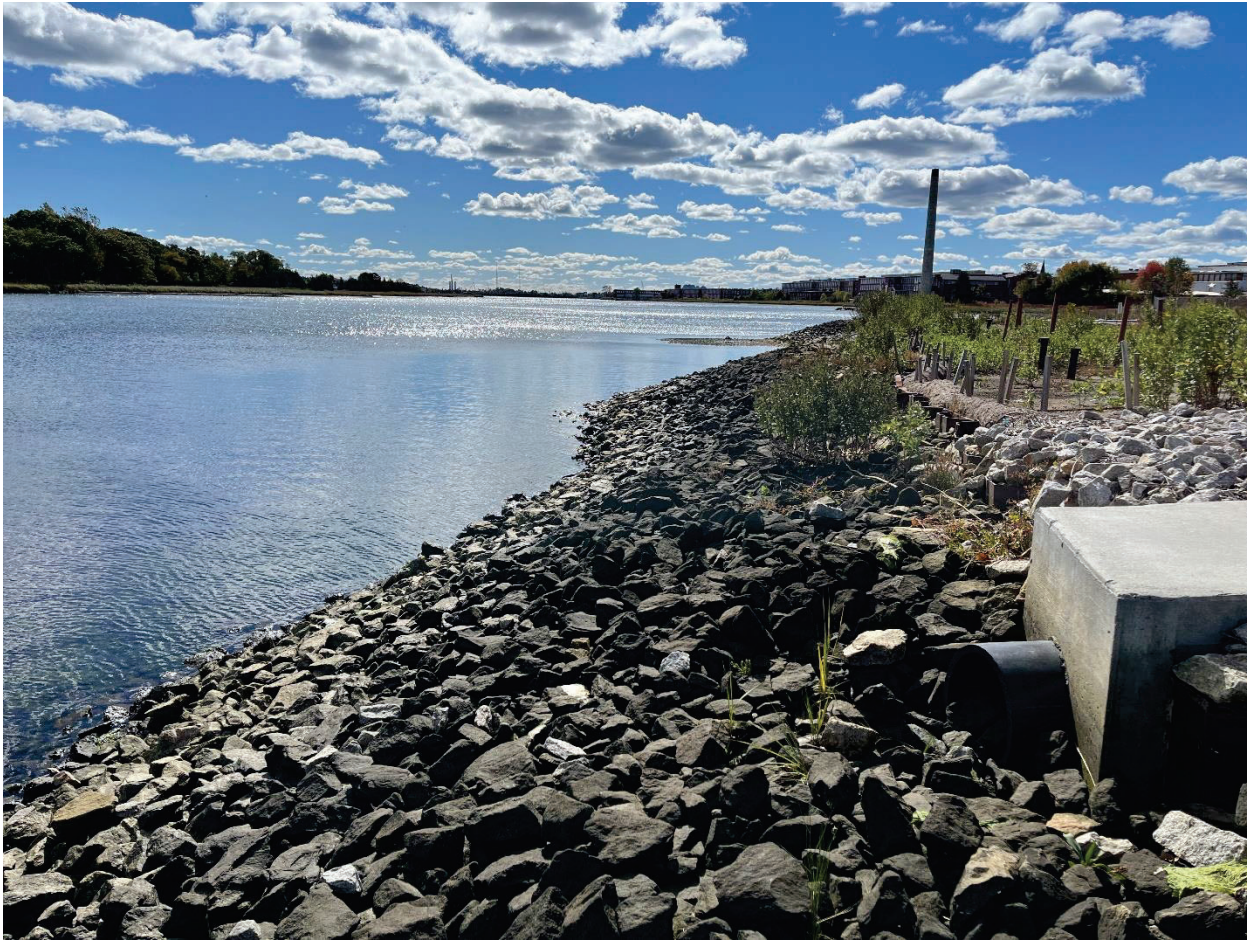
Figure 4: Aerovox Cap: Looking south showing the South Trench storm drain outlet in the foreground.
