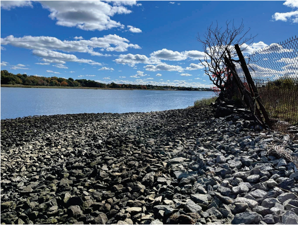
Figure 8: Crib Cap: Looking south showing the top of the abutting seawall with chain link fence along the western side of the cap.
