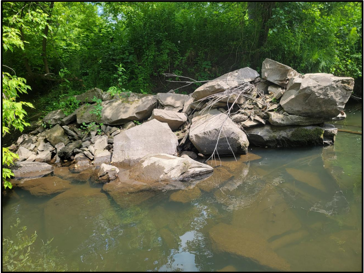
Figure A-11. RF#5, Abutment 1: A bridge abutment composed of medium and large cut stones with smaller rocks used as fill between the larger stones. Located on the western bank.
