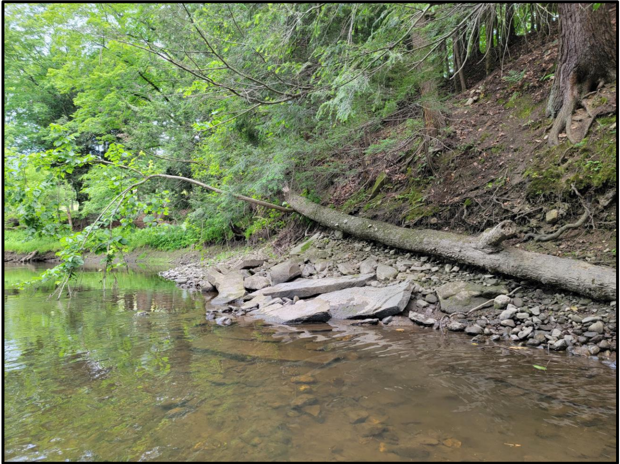
Figure A-14. RF#7: Multiple very large cut tabular cut rocks located along the eastern bank. The cut rocks are roughly 4 to 5 meters long and 1 to 2 meters wide. Among the cut rocks are small to medium cobbles and sub-angular rocks. The eastern bank is very steep and has a coniferous vegetation.
