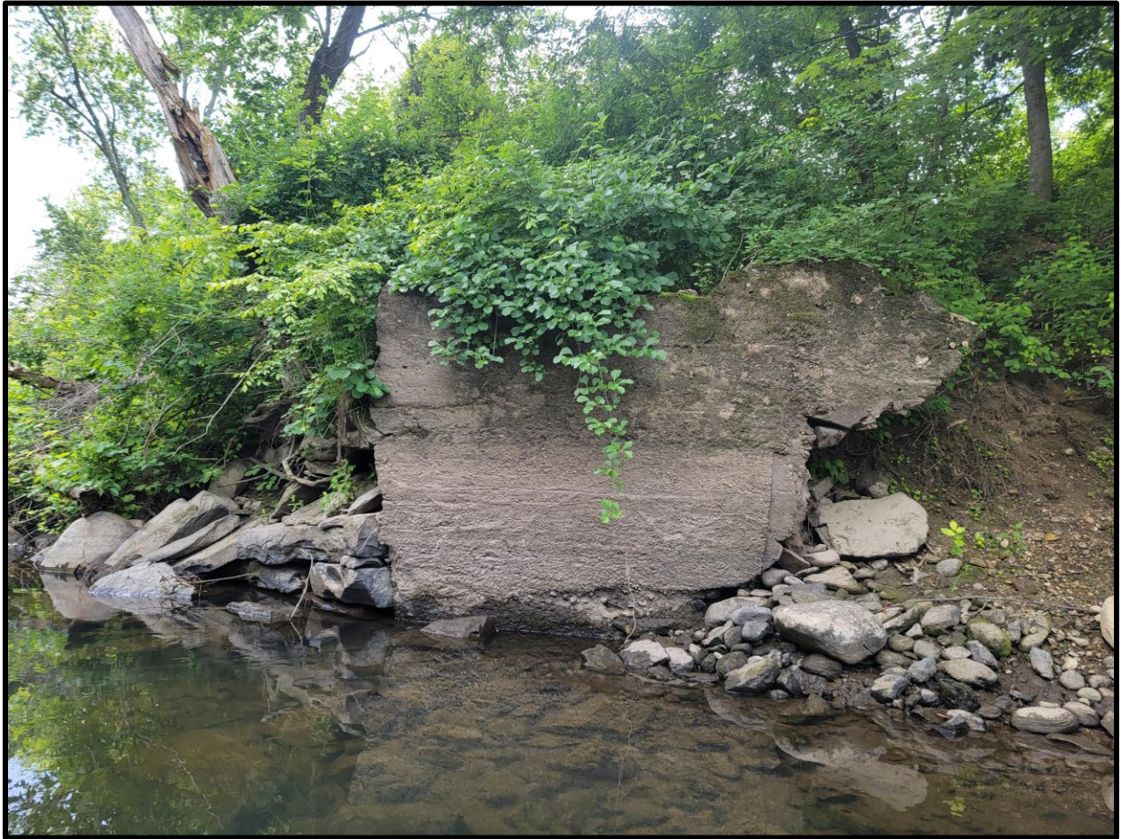
Figure A-15. RF#8, Abutment 1: A bridge abutment composed of medium to large cut stones with a concrete mixture used as mortar between the stones. One of the sides is faced with the concrete mixture. The concrete mixture includes small angular rocks, rounded rocks, and coarse sand. Located on the western bank. Dimensions: height = 2 meters; width = 2.5 meters.
