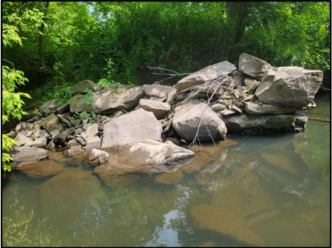
Figure A-12. RF#5, Abutment 2: A bridge abutment composed of small and medium cut stones, much of which is obstructed by thick vegetation. Located on the eastern bank.
