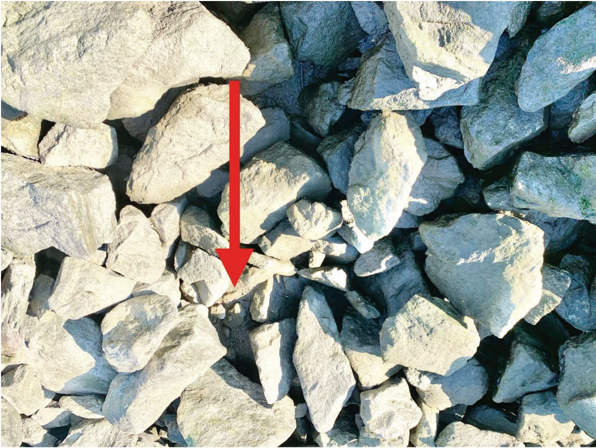
Figure 12: Crib Cap: showing a very small area needing additional armor stone.
