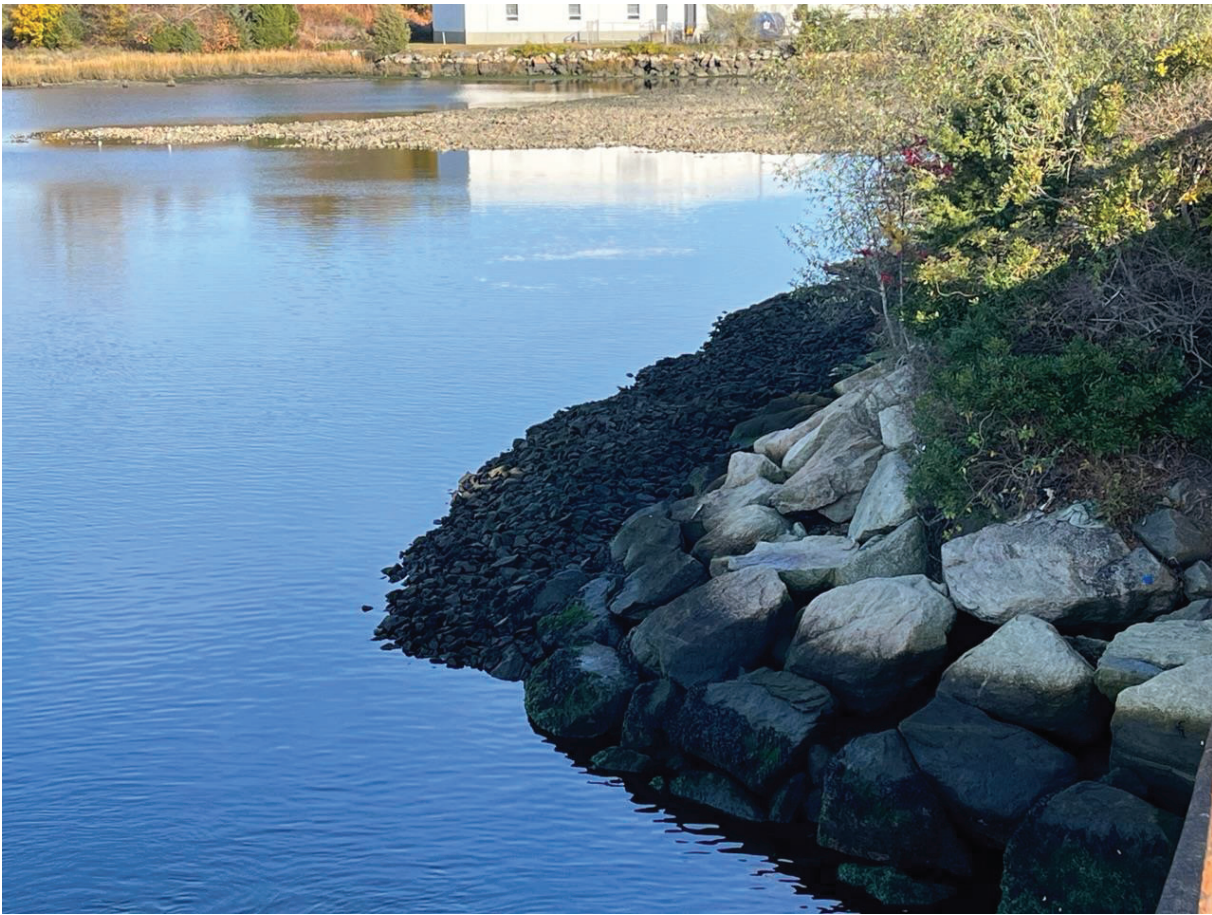
Figure 23: Cogg-East Cap: looking east showing the western edge of the cap at the Coggeshall St bridge opening. Cap armor stone also shown in background.
