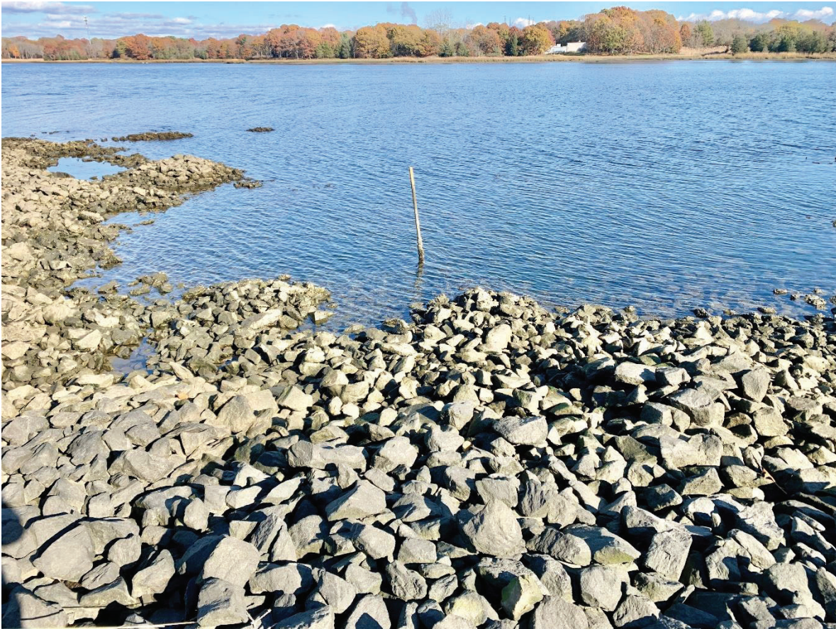
Figure 9: Crib Cap: Looking northeast showing area near a drainage outfall (possibly defunct).
