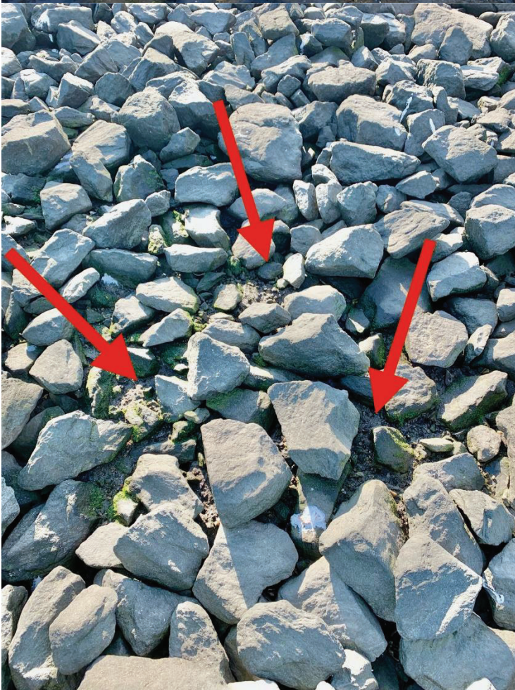
Figure 18: Pilot CDF Shore- line Cap: showing area with thin armor stone layer and some exposed sand isolation layer.
