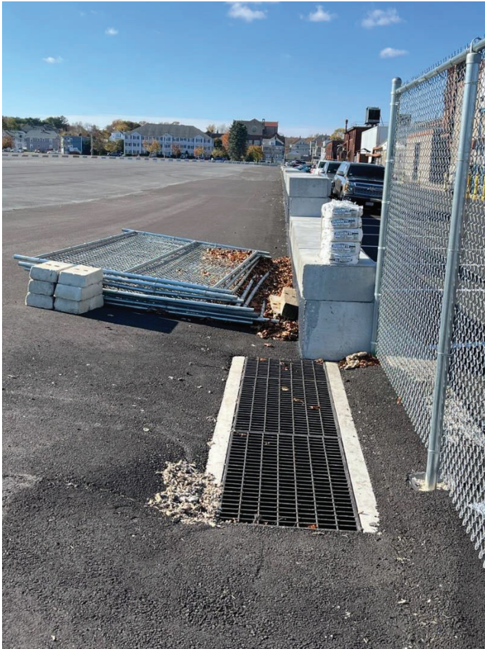
Figure 3: Aerovox Cap: Looking west showing the as- built condition of the recently completed (summer 2023) North Trench drainage grating.
