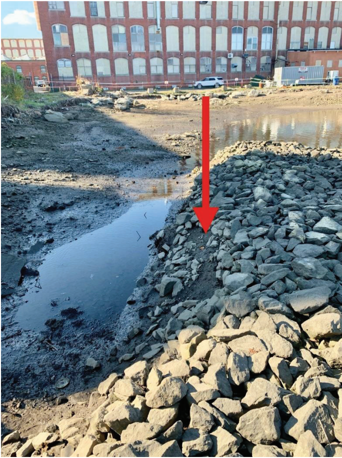
Figure 11: Crib Cap: Looking west showing an area needing additional armor stone at the northwestern end of the cap.
