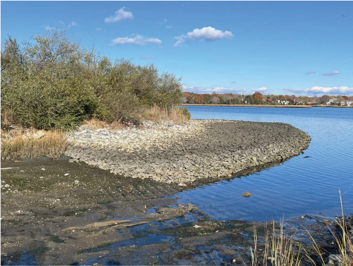
Figure 17: Pilot CDF Shore- line Cap: looking northeast showing the southern edge of the cap. Toe of slope remains well defined.
