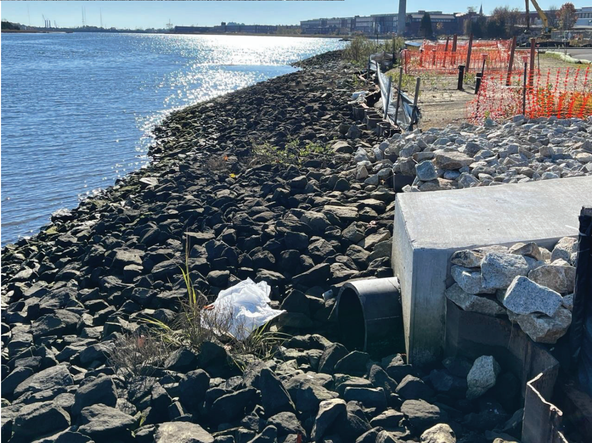
Figure 4: Aerovox Cap: Looking south showing the South Trench discharge structure in foreground. Emergent salt grass noted in previous inspections remains near the outfall (the void spaces in the armor stone are likely filling in with silt from the drainage discharge).
