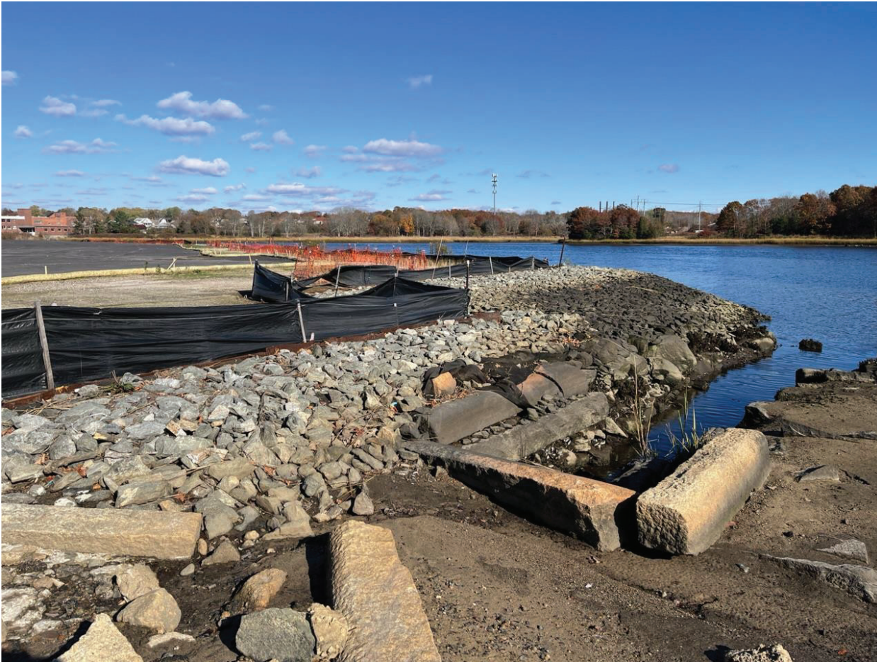
Figure 7: Aerovox Cap: Looking northeast showing the southern section of the cap and the abutting Hadley Street storm drain
