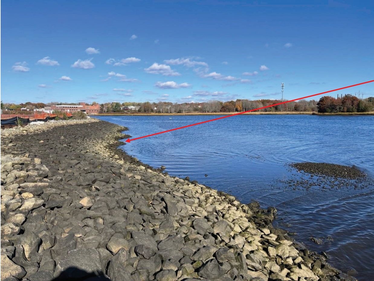
Figure 6: Aerovox Cap: looking north showing a serrated pattern at the waterline in some areas.
