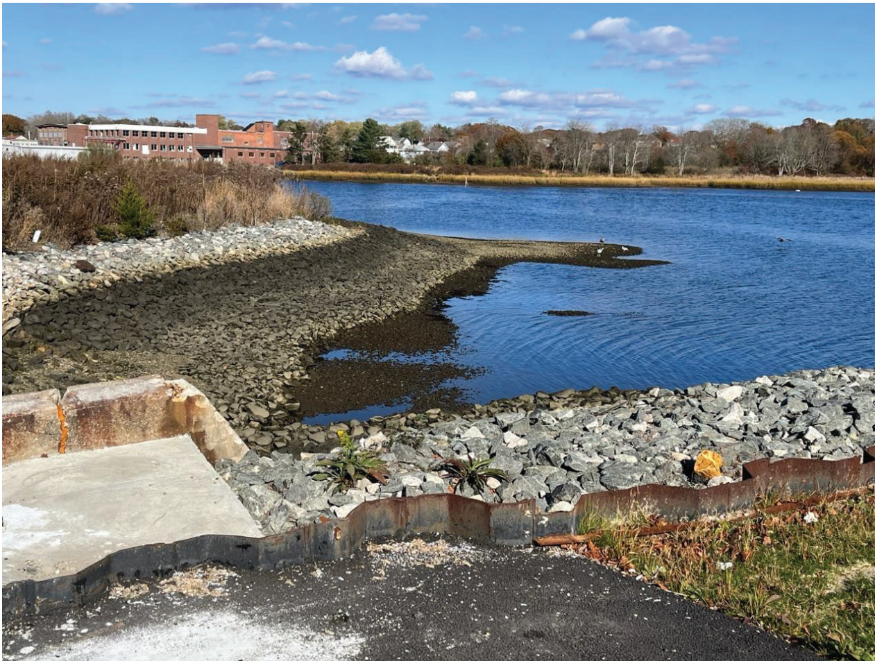
Figure 2: Aerovox Cap: Looking NE showing “capacitor cove.” The lower edge of the larger armor stone on the river bank can be seen where it meets the smaller armor stone of the flatter portions of the cap.
