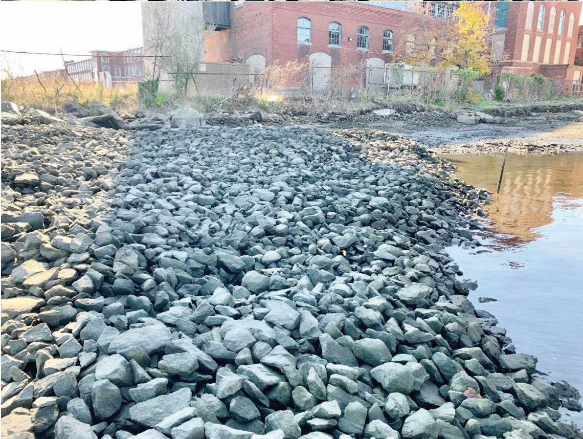
Figure 10: Crib Cap: Looking southwest showing the northern edge of the cap. The southern edge of the ongoing WZ2/3 shoreline excavation can be seen in the background.
