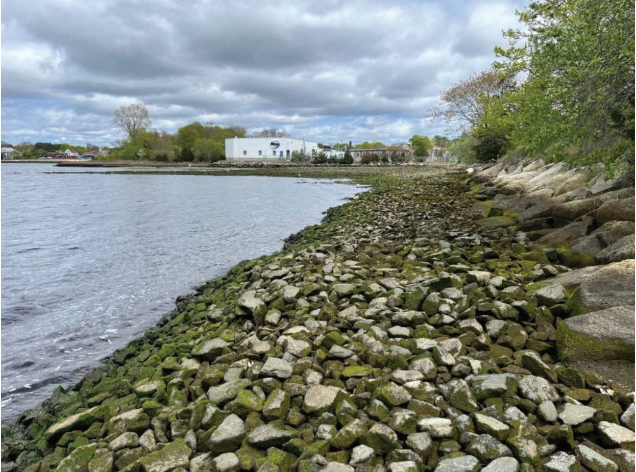
Figure 18: Coggeshall- East Cap looking east. Photo taken from near the bridge opening.
