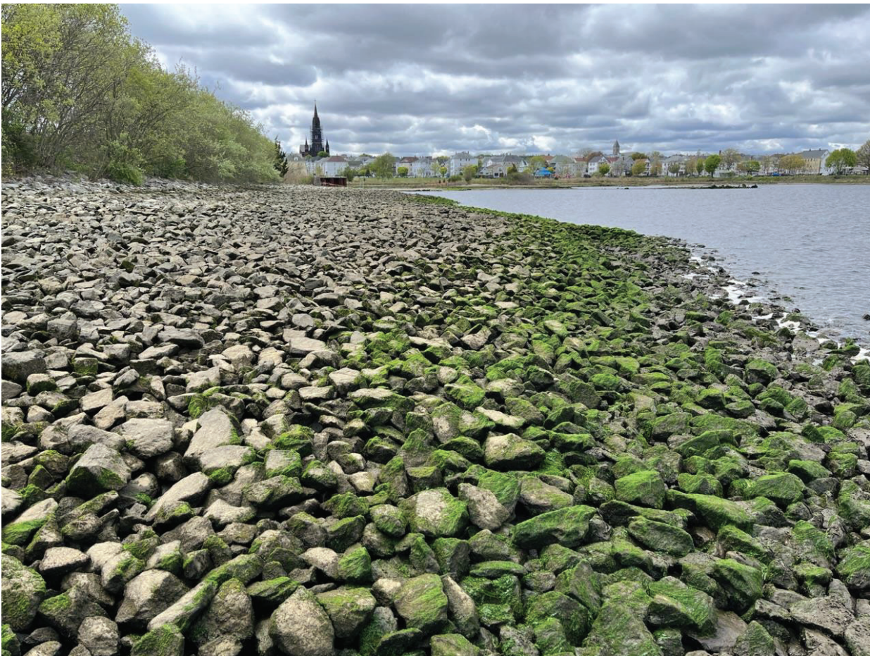
Figure 14: Pilot CDF Cap looking west, showing the northern edge of this cap.
