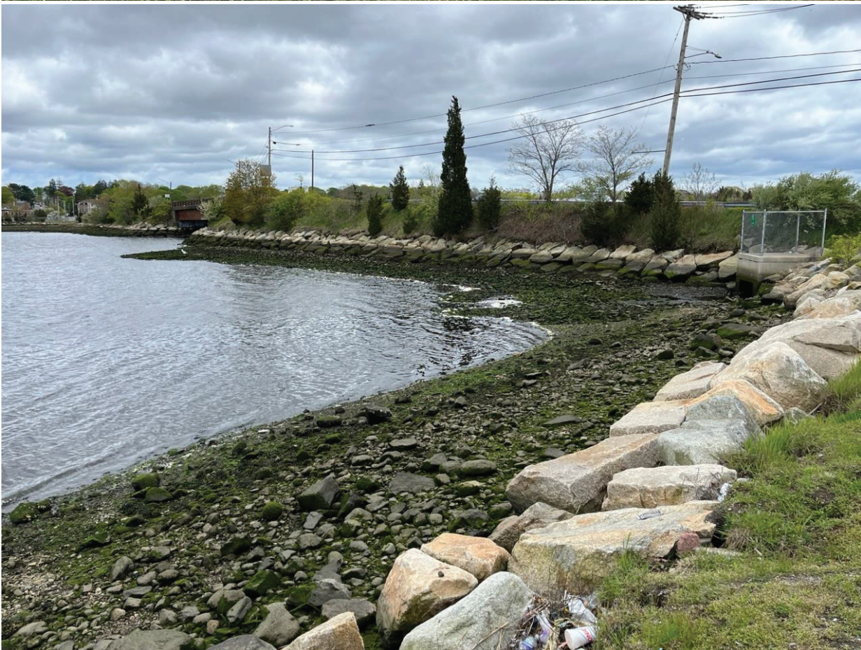
Figure 16: Coggeshall- West Cap looking SE. City storm drain structure is located at the 90 degree turn of the shoreline.
