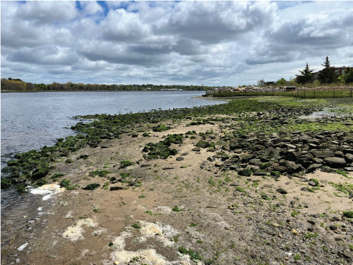
Figure 11: L-014 Cap looking south, showing silt deposition within the stone cap surface.
