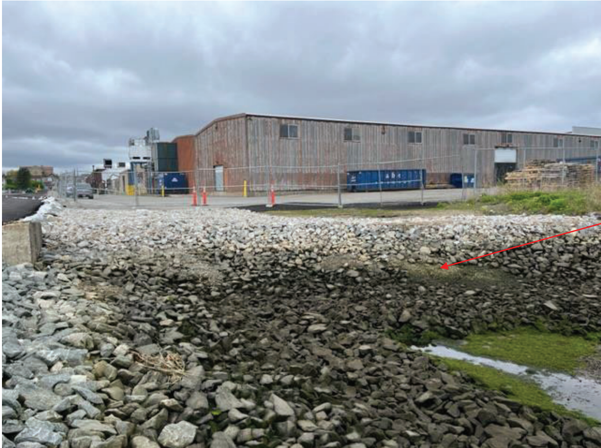
Figure 2: Aerovox Cap: Looking west showing the improved east end of the Graham Street drainage swale, with larger stone added. Remnants of the original smaller stone that washed out can be seen.
