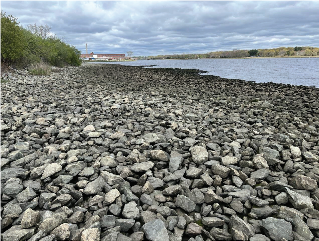
Figure 13: Pilot CDF Cap looking north, showing the eastern edge of this cap.
