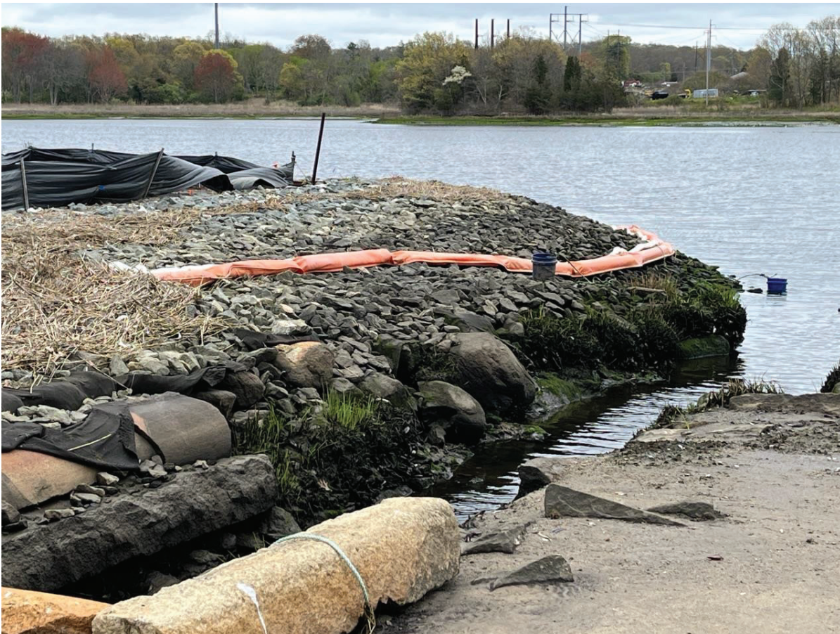
Figure 5: Aerovox Cap: Looking NE showing the Hadley Street storm drain outfall which abuts the southern end of this cap.
