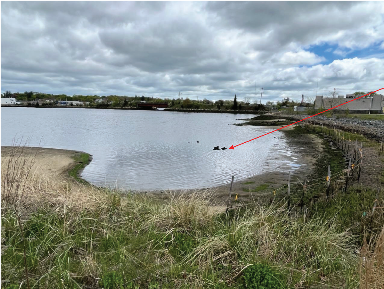
Figure 15: Parcel 265 Cap looking east. Only a few cap stones are visible at low tide at this cap.
