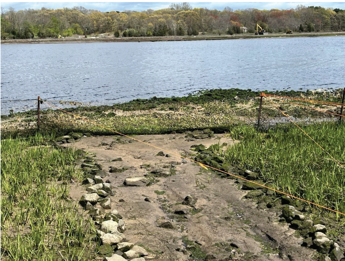
Figure 10: L-014 Cap looking east, showing the WZ-4 drainage swale and related silt and topsoil deposition.
