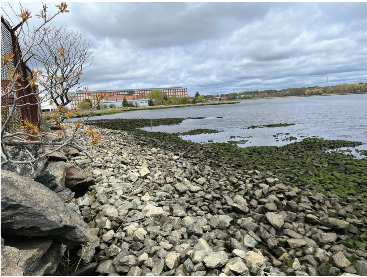
Figure 6: Crib Cap looking north. The white stake is the location of an old storm drain.
