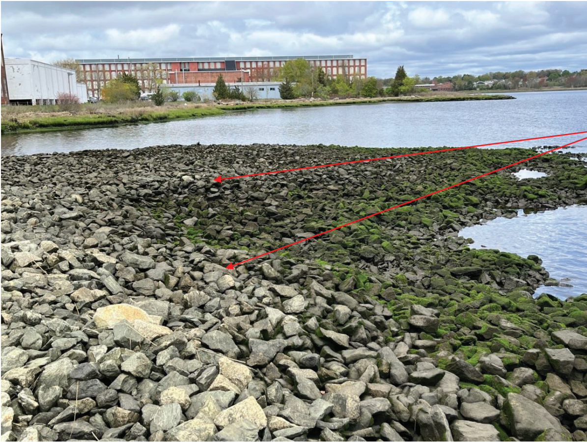
Figure 7: Crib Cap looking north, showing examples of high spots to be smoothed per the one action item discussed above on p.1.
