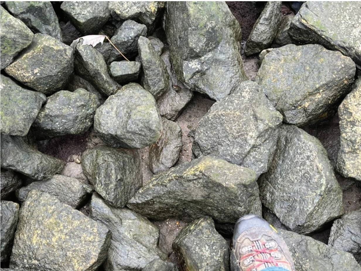
Figure 10: Crib cap showing very small area of exposed sand (app. 2 sq ft) 20-25' south of the white pole noted in Figures 7 and 8 above.
