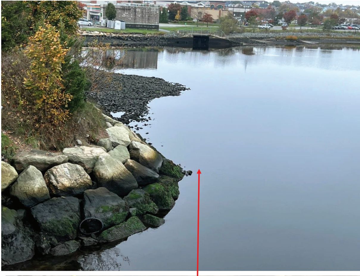
Figure 19: Cogg-West Cap looking west from the bridge opening. Shoreline outfall structure in the background (with chain link fence) is the relocated Sawyer Steet CSO.
