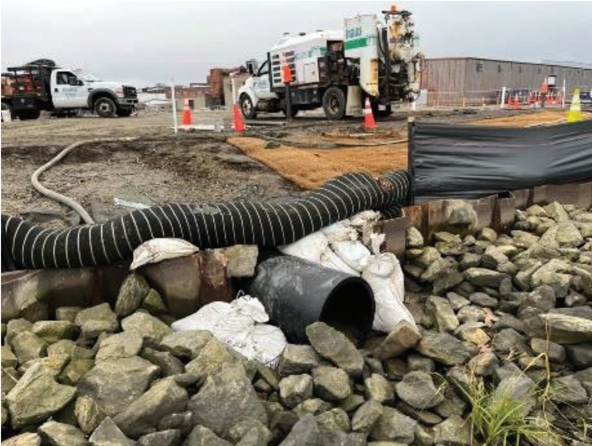
Figure 5: Aerovox cap looking northwest showing the new south trench outfall. This former trench will now be an HDPE pipe covered with concrete (with similar invert elevation). Note marsh grass ( Spartina alterniflora? ) emerging in foreground.
