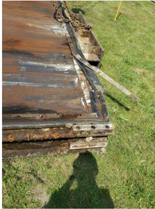
Photo 9: Top seal of gate prior to replacement. Note displaced seal.
