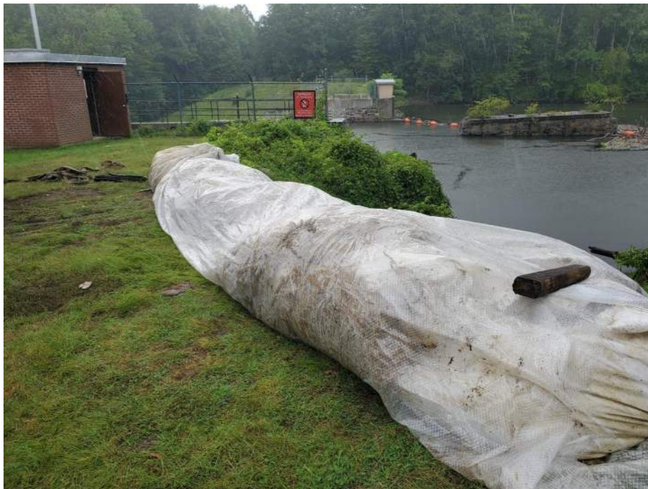
Photo 14: Plastic wrapped sheeting and sandbags pending proper disposal.
