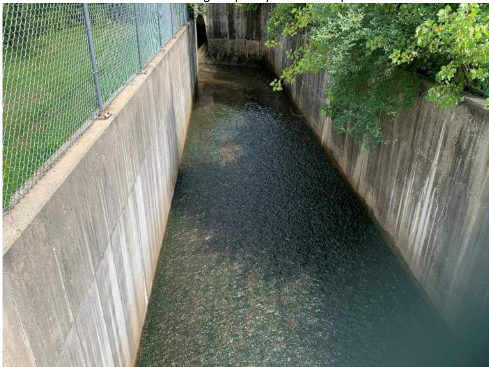
Photo 6: Temporary bulkhead leakage flow at tailrace prior to placing sandbags and plastic sheeting.
