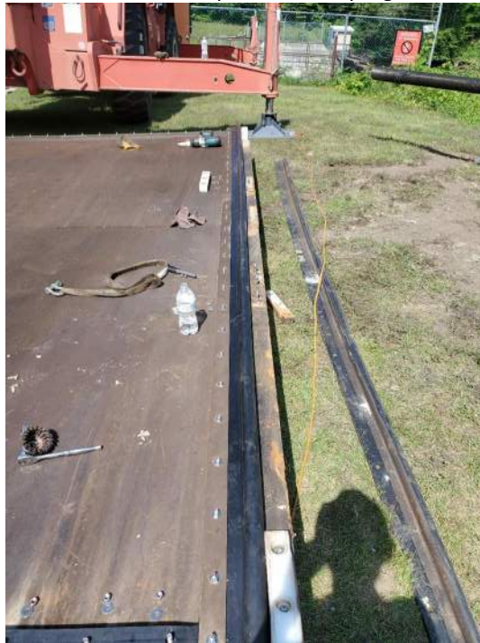
Photo 12: Seal replacement in progress.
