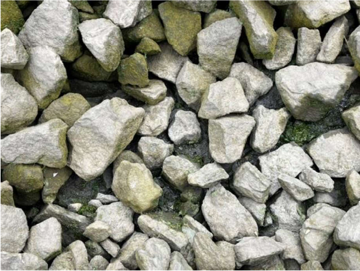
Figure 7: Crib cap showing the small areas of exposed sand needing addition of armor stone.
