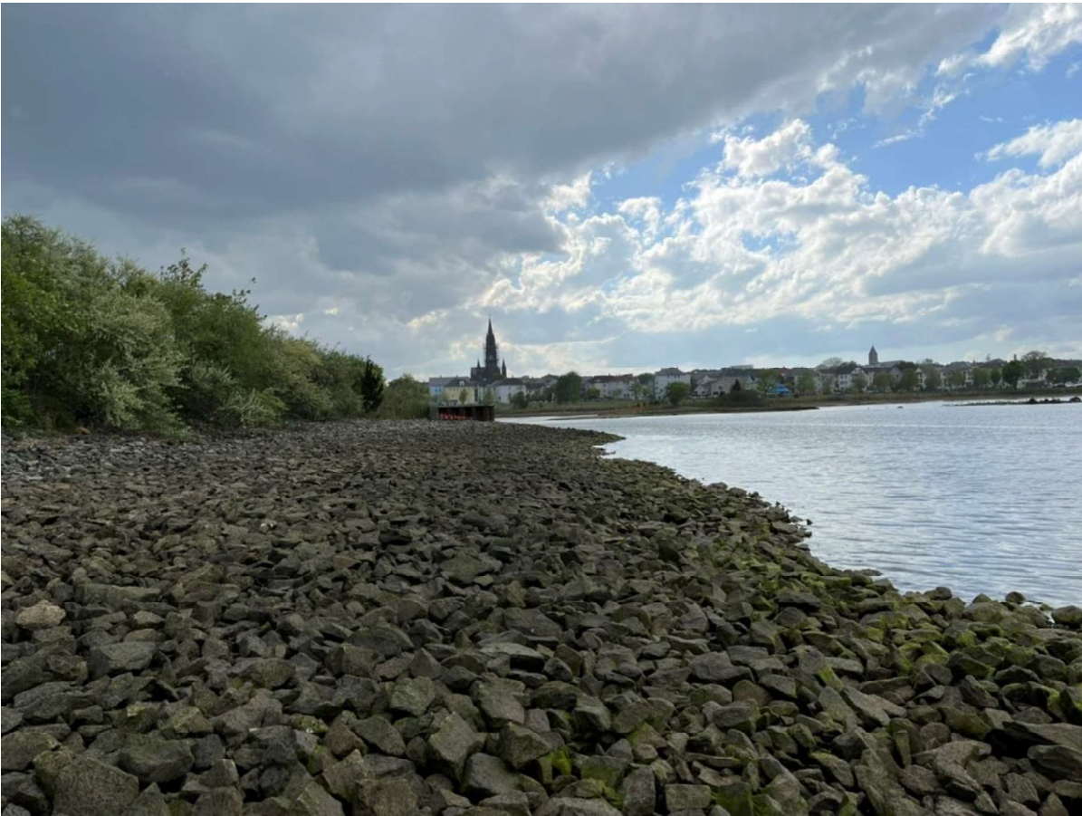
Figure 15: Pilot CDF shoreline cap looking west showing the northern E/W-trending portion of the cap.
