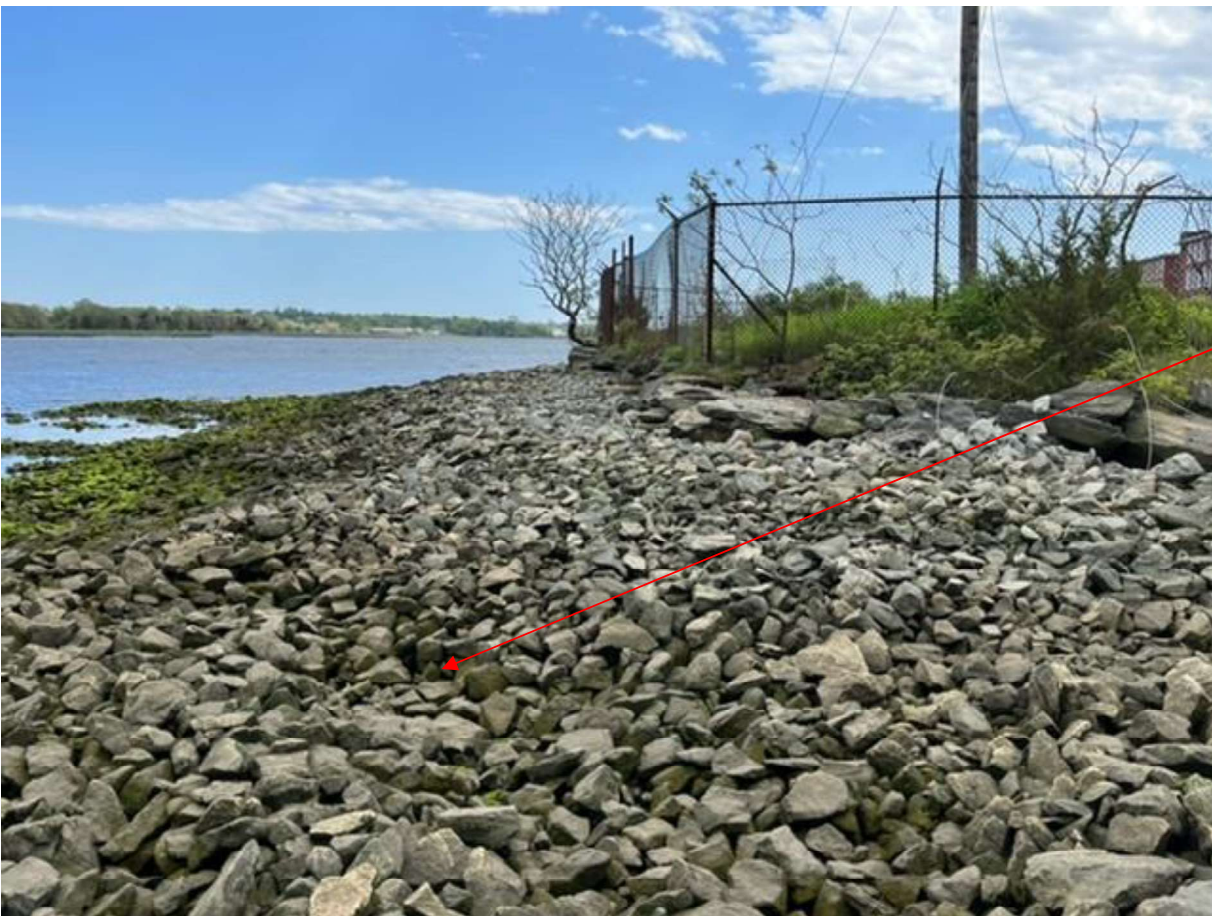
Figure 6: Crib cap looking south showing the small area needing addition of armor stone (see Figure 7 for closeup).
