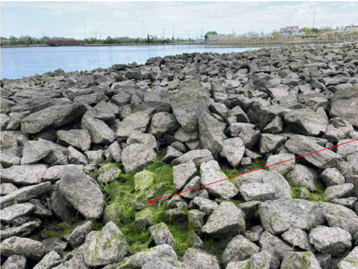
Figure 14: Pilot CDF shoreline cap looking south showing small area needing additional armor stone (area covered with green algae).
