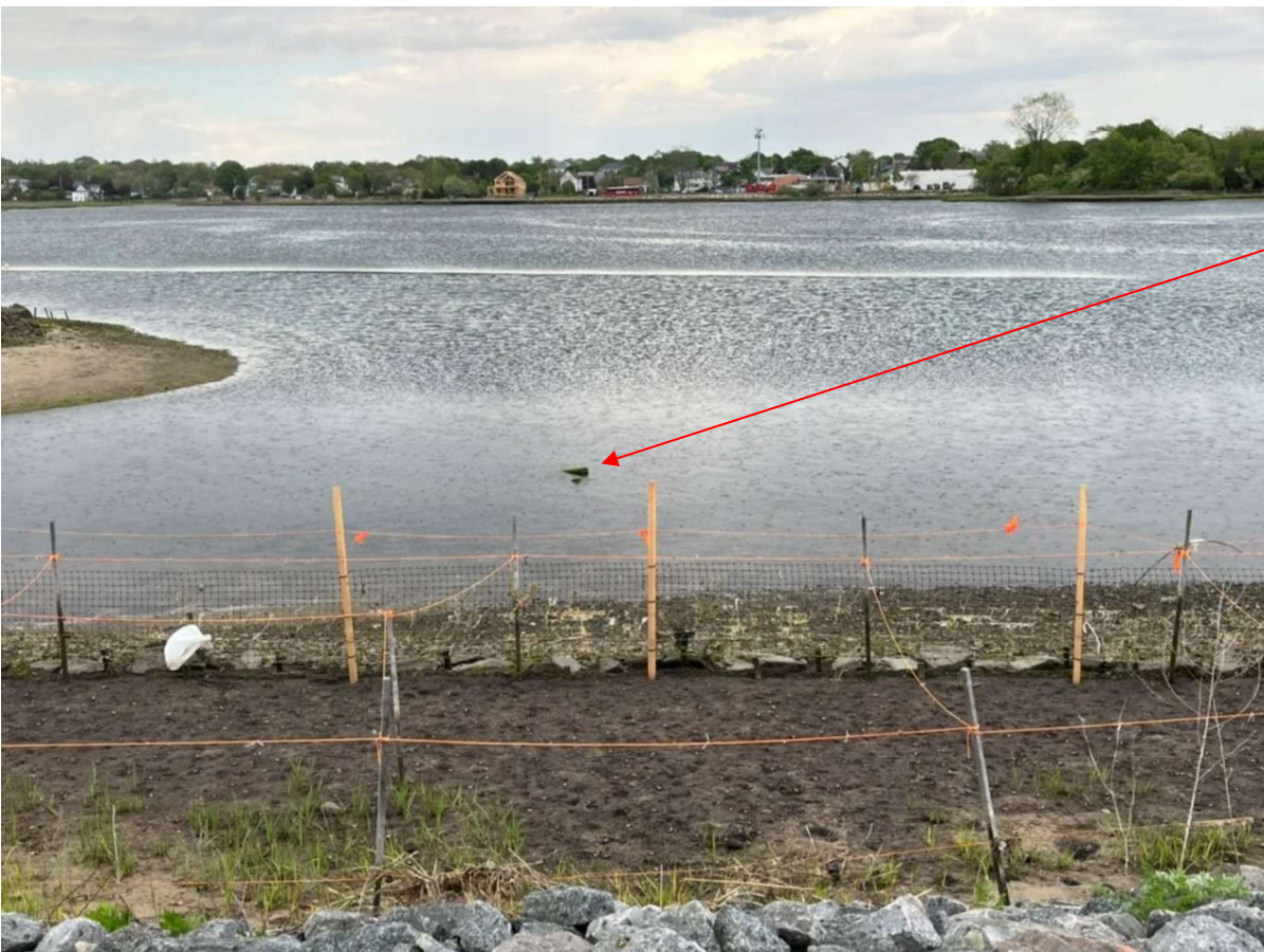
Figure 16: Parcel 265 cap looking east. Only the very top of the stone cap can be seen. The repaired parcel 265 herbivory fence can be seen in the foreground.
