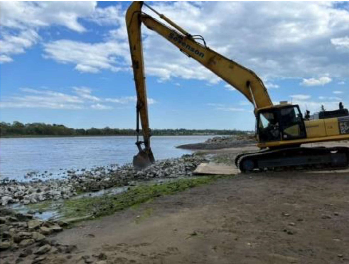
Figure 9: L-014 cap looking south. Additional armor stone being added by the WZ 4 intertidal crew to create a more uniform surface to aid in visual inspections moving forward.
