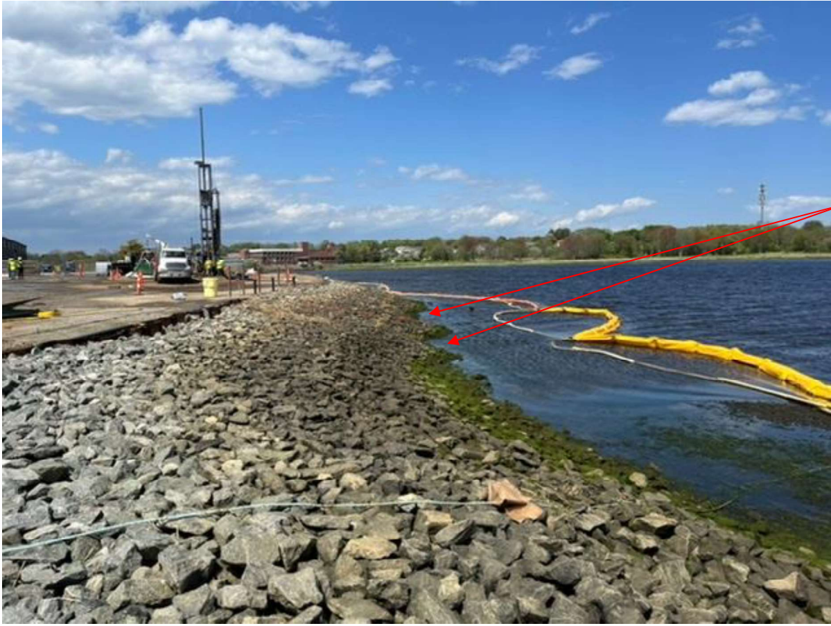
Figure 3: Aerovox cap looking north along the landward/western edge of the cap. Note the serrated pattern developing at the toe of slope.
