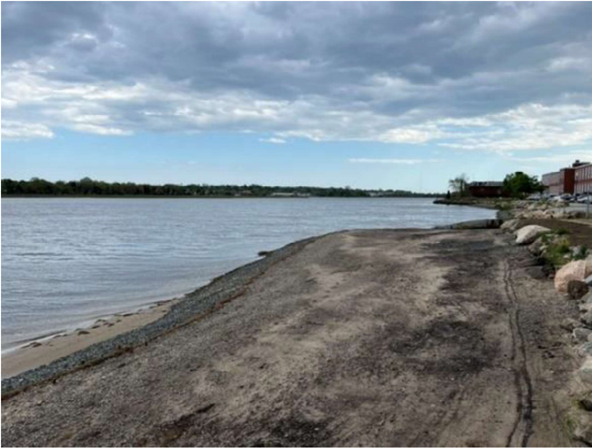
Figure 11: L-114 cap (fully submerged, not visible). This photo shows the recently repaired WZ4 intertidal area, ready for saltmarsh plantings. Note coir log and gravel wedge at the seaward face of the low marsh planting area.
