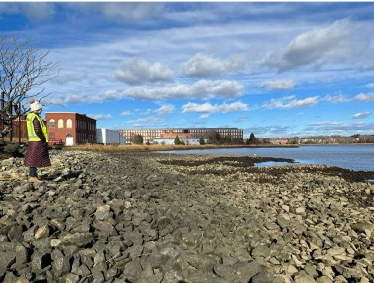
Figure 10: Crib cap looking north. White stake in middle is a stormwater outfall (see Figure 12).
