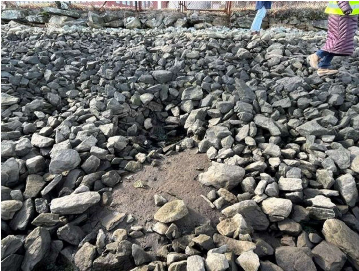
Figure 11: Crib cap showing the small area in need of armor stone.
