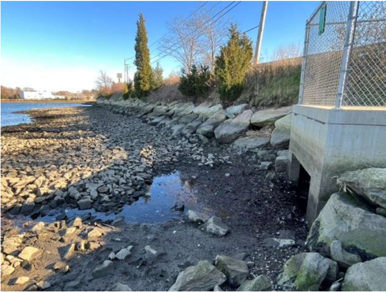
Figure 23: Cogg-West cap looking east along bridge embankment. City storm drain in foreground.
