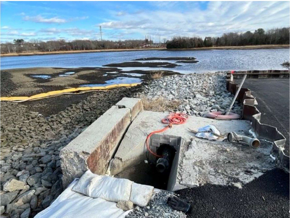
Figure 4: Aerovox cap looking east showing the North Trench storm drain (plugged as part of 21E cleanup).
