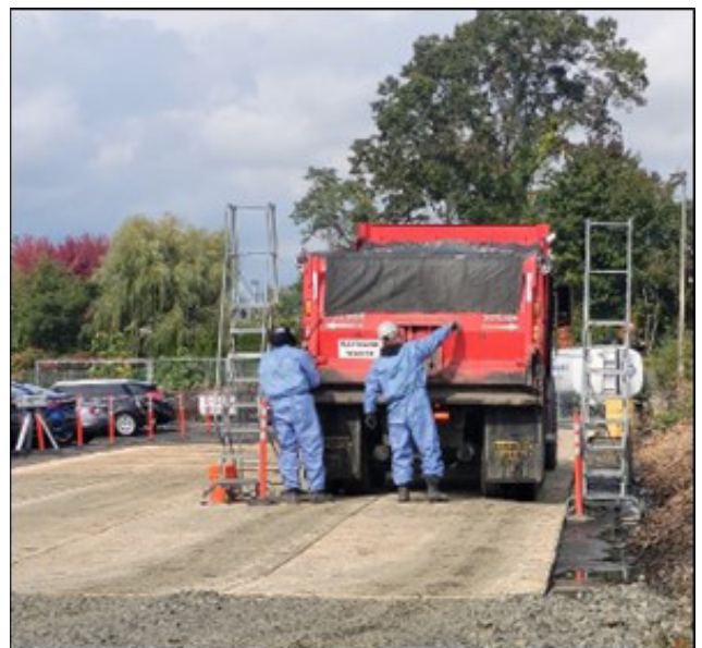
Example of secured truck used at the Raymark Superfund Site in Stratford, Connecticut
