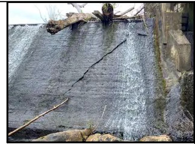
PHOTO 1 - DOWNSTREAM DIAGONAL CRACK
