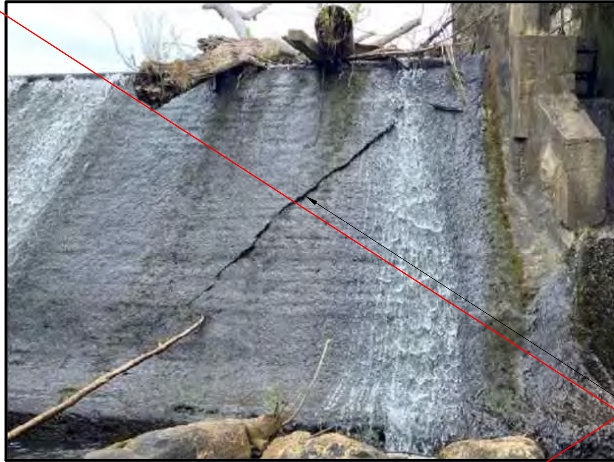
REPOINT DOWNSTREAM DIAGONAL CRACK NOT TO SCALE
