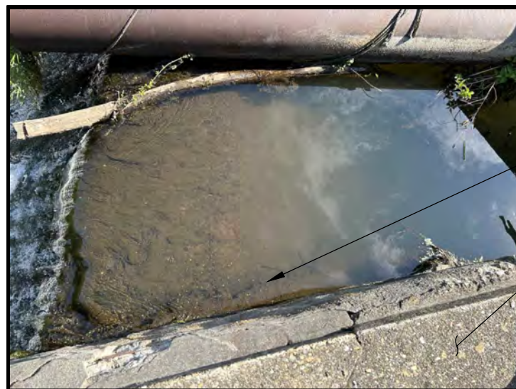
PHOTO 3 - EXISTING CONDITIONS CONCRETE SURFICIAL CRACK/VOID NOT TO SCALE
