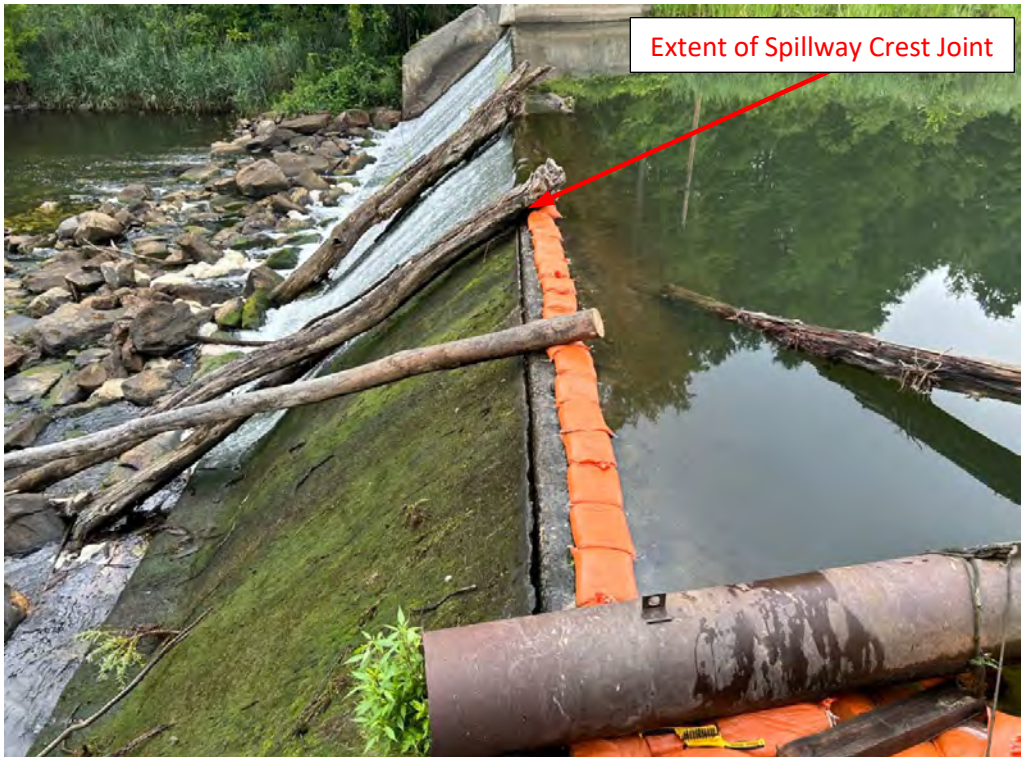
Photo 5. Spillway crest joint before repairs; extent determined by probing.
