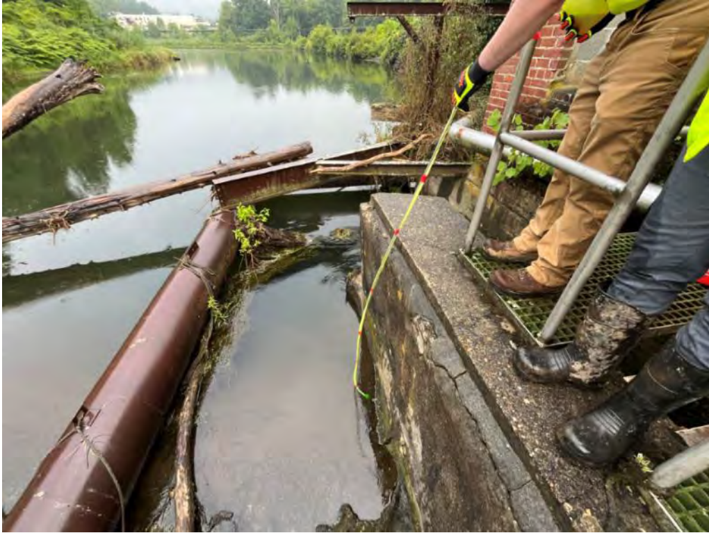
Photo 1. Introducing tracer dye into the crack/void at the former vortex location.
