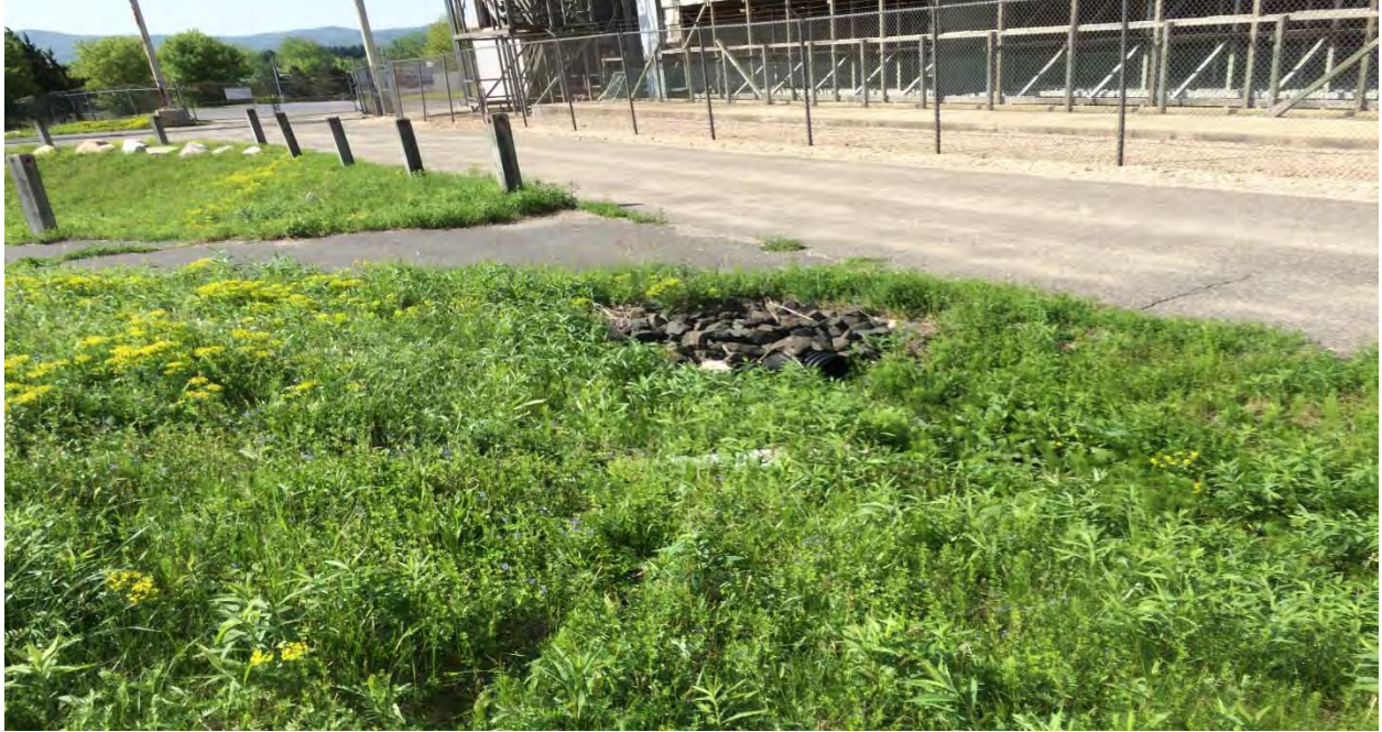
Photo #11: View of drainage ditch along southern edge of Building 71 OPCA (photo direction East).
