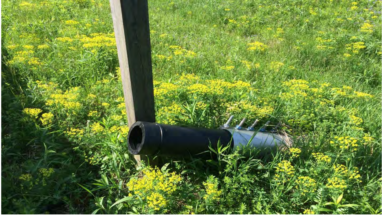
Photo #7: View of leachate collection cleanout pipe of the Building 71 OPCA (photo direction South).
