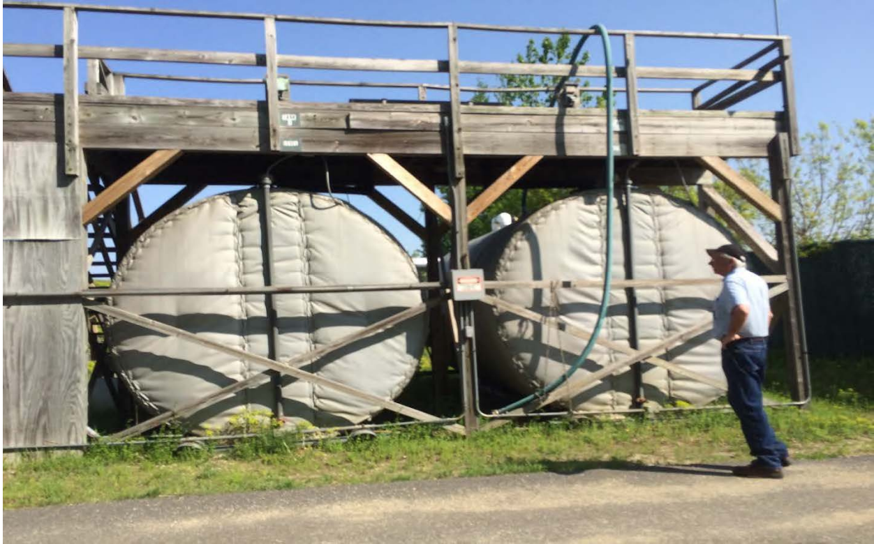
Photo #9: View of leachate collection tanks (photo direction West).
