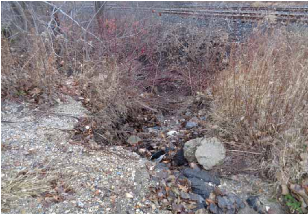
Photo #4: Erosion present on Parcel L12-1-101.
