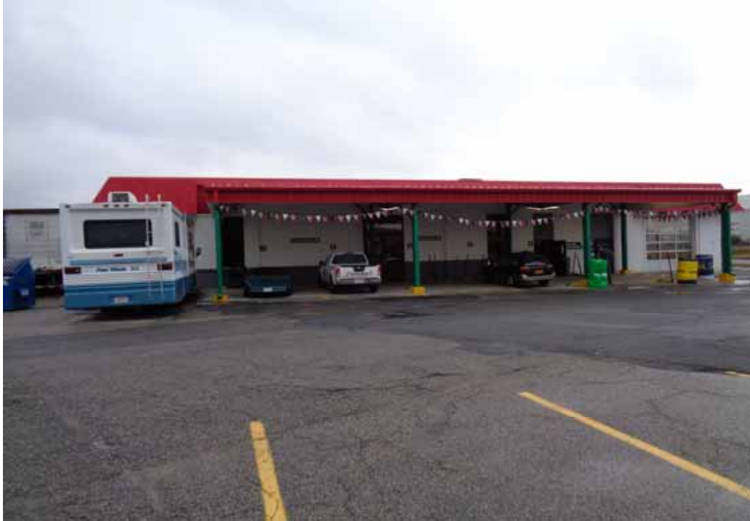
Photo #1: Completed installation of eight concrete foundation footings and installation of a concrete pad on Parcel L12-1-4.
