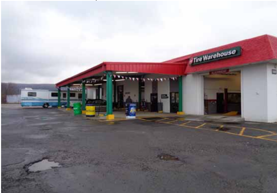
Photo #2: Completed installation of eight concrete foundation footings and installation of a concrete pad on Parcel L12-1-4.
