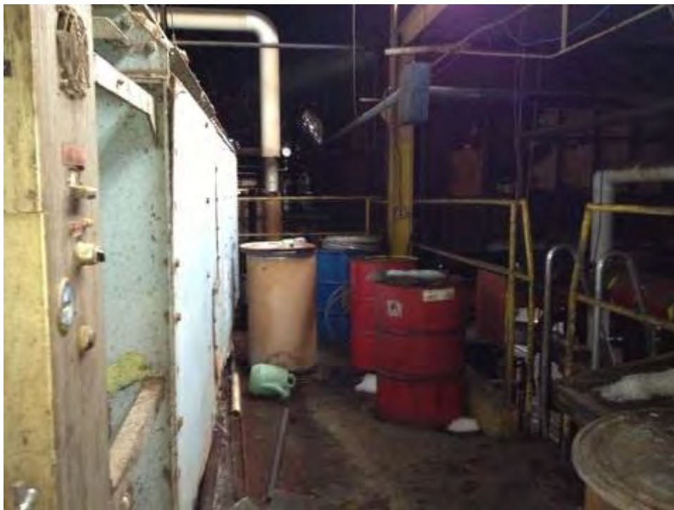
SCENE: View of empty drums in the southeast corner of the second floor mezzanine.
