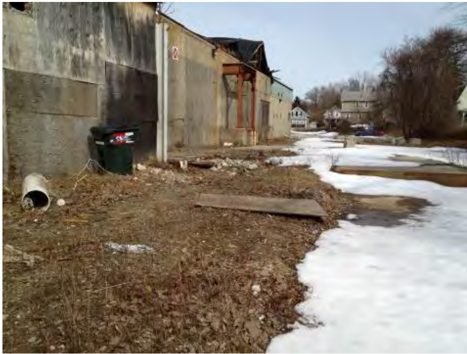
SCENE: View of the south side of the building. Photograph taken facing northeast.
