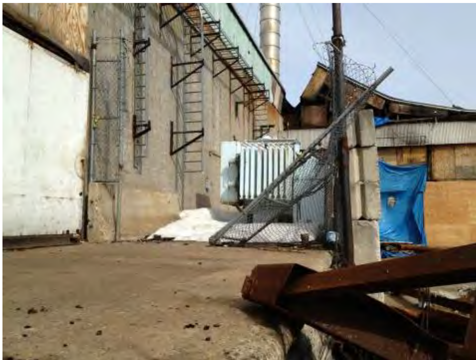
SCENE: View of the transformers on the southeast loading dock. According to the property manager, the transformers are scheduled for removal and disposal. Photograph taken facing east-northeast.
