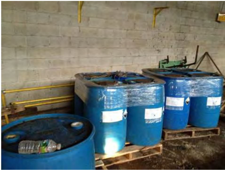
SCENE: View of drums of Ferric Sulfate, staged adjacent to the Caustic tank.
