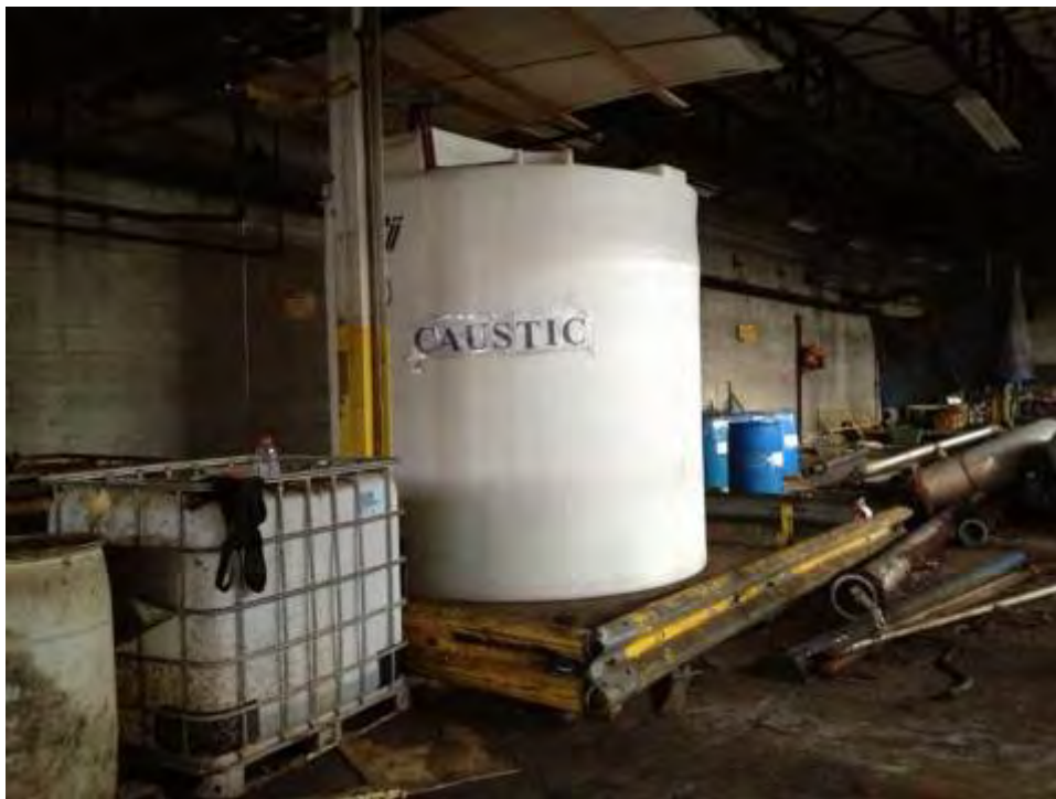
SCENE: View of the Caustic tank, with unlabeled containers to the left, and drums of Ferric Sulfate to the right.
