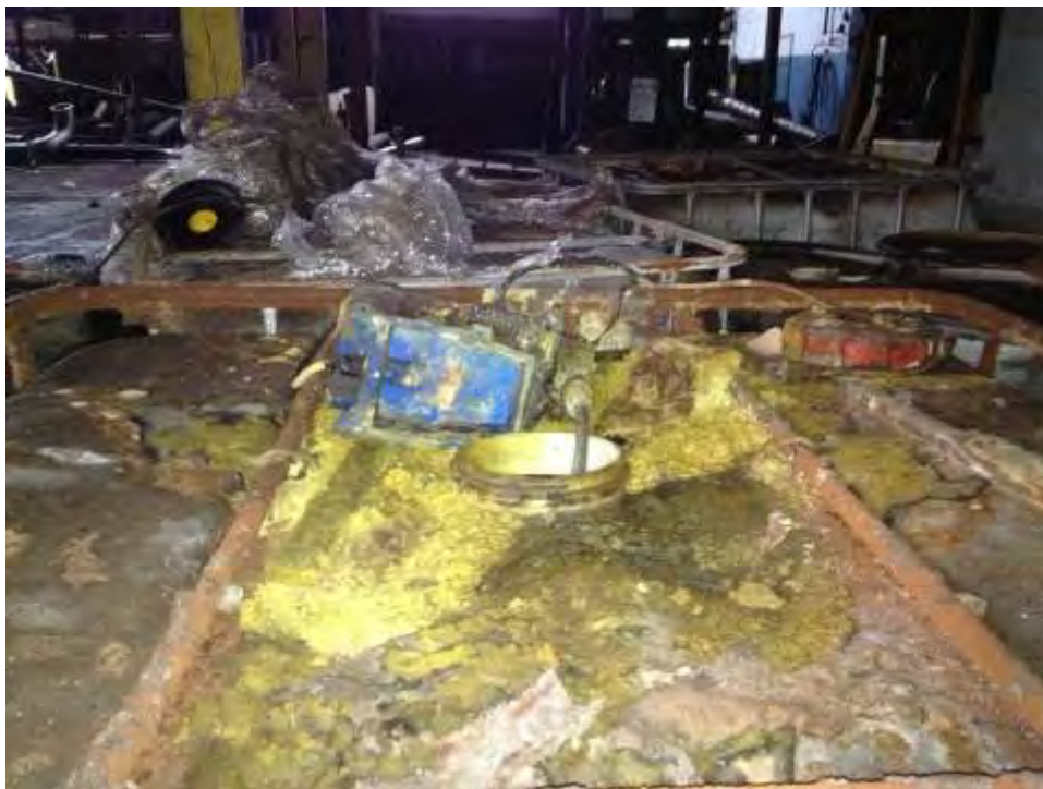
SCENE: View of yellow crystals around the opening of a tote that was located adjacent to the Caustic tank.
