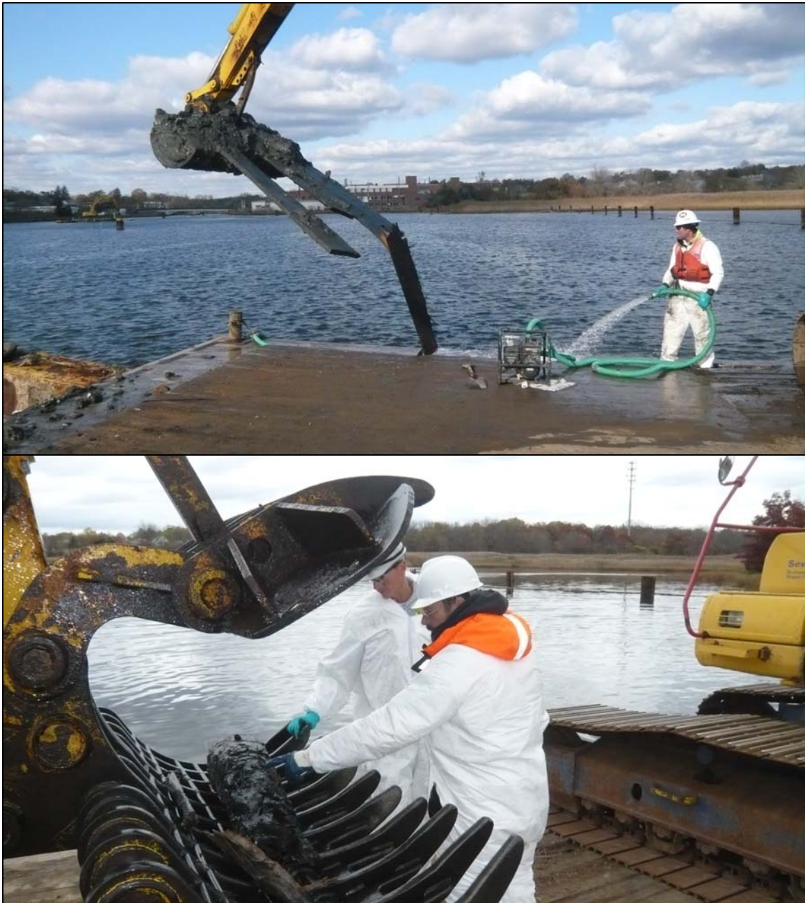
Figure 2-2. Systematic debris removal and ship timber recovery were conducted within the unanticipated shipwreck discovery study area in November 2009 under the supervision of the project archaeologist, David Robinson (bottom image) (top photograph by David Robinson; bottom photograph by Josh Cummings).
