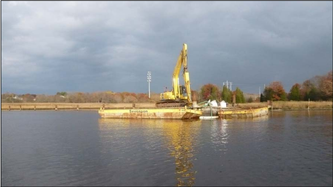
Figure 2-1. NBHSS debris removal spud-barge with machine and hopper barges (one for the recovered timbers and the other for miscellaneous debris) positioned over the unanticipated shipwreck discovery location in November 2009 (photograph by David Robinson).
