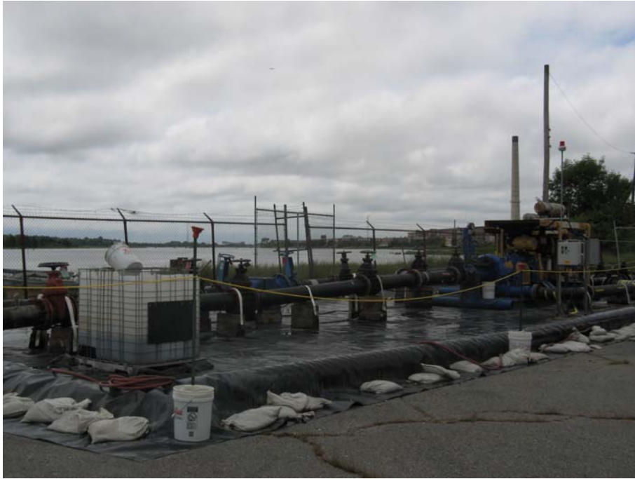
Photo 11: Booster Pump area
