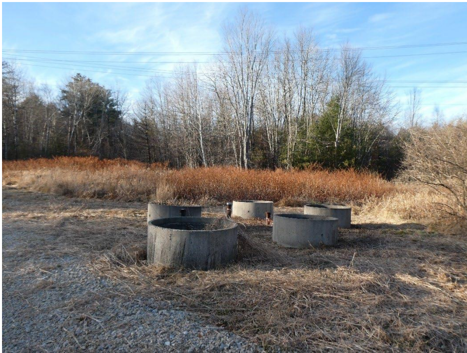
Concrete protection around wells
