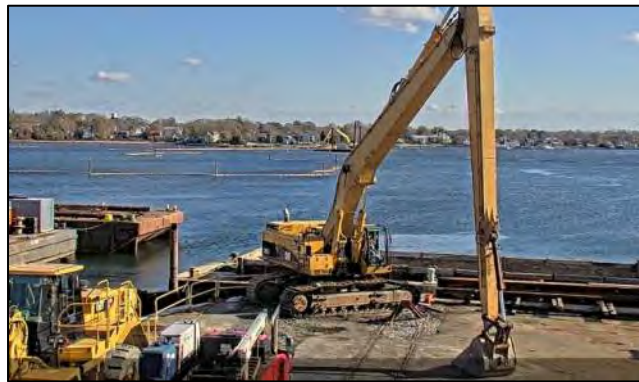
Landside excavator waiting on next deck barge. Dredge PC-1250 dredging at CAD Cell #4 in background.
