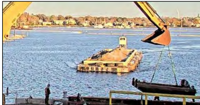
Tug bringing loaded deck barge to North Terminal area for cofferdam cell #1 filling.
