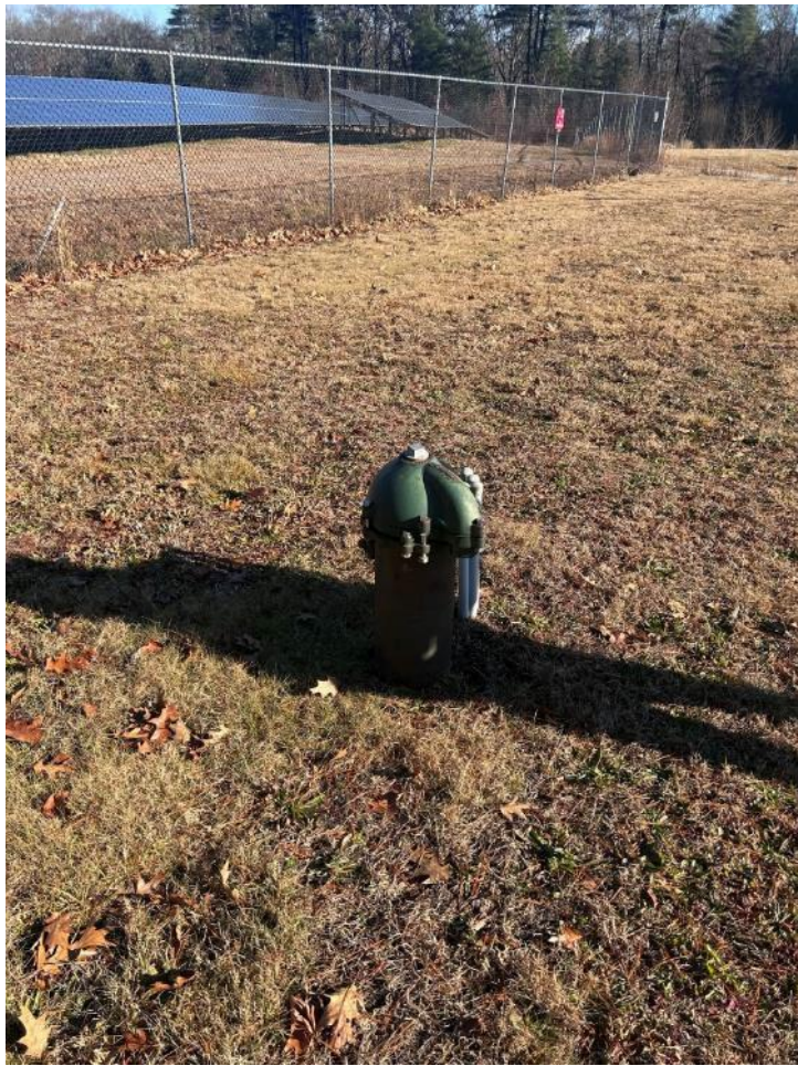
Inactive pumping well on Concord Bus Facility
