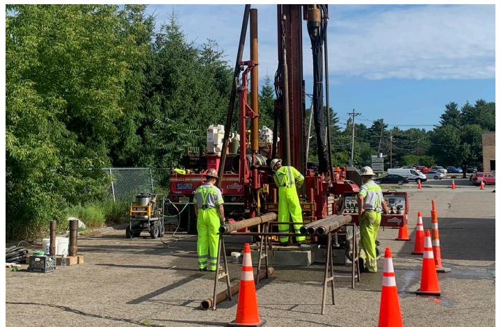
A drilling crew advances a bedrock boring on private property in South Wilmington in August 2022. Groundwater investigations on and off the Olin property continue under a 2007 legal agreement between EPA and the Potentially Responsible Parties ("PRPs").
