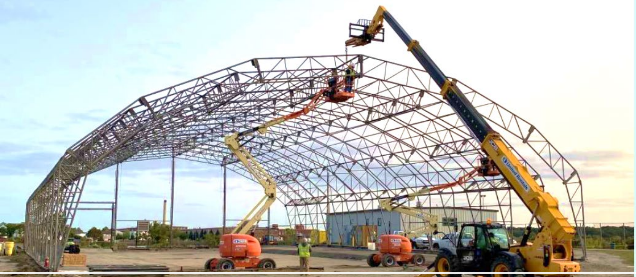
Deconstruction and Transfer of the Sawyer Street Desanding Facility to the City of New Bedford September 2020
