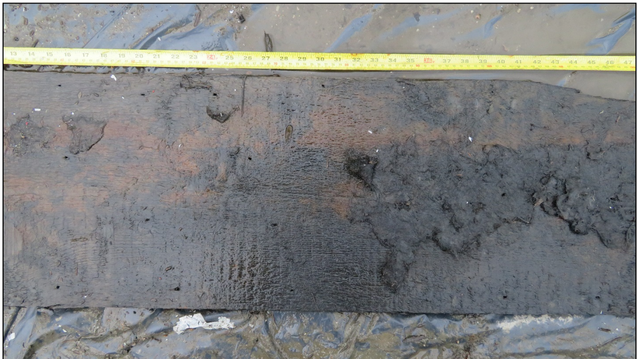
Figure 19. Irregularly angled, widely-spaced, saw kerf marks were visible on both sides of the sheathing (top and bottom images), and were consistent with hand-cut “pit-” or “platform-” sawn lumber. Large areas of intact tarred felting were also still visible adhering to the inboard surfaces of the wood hull sheathing (photographs by David S. Robinson, DSRA).
