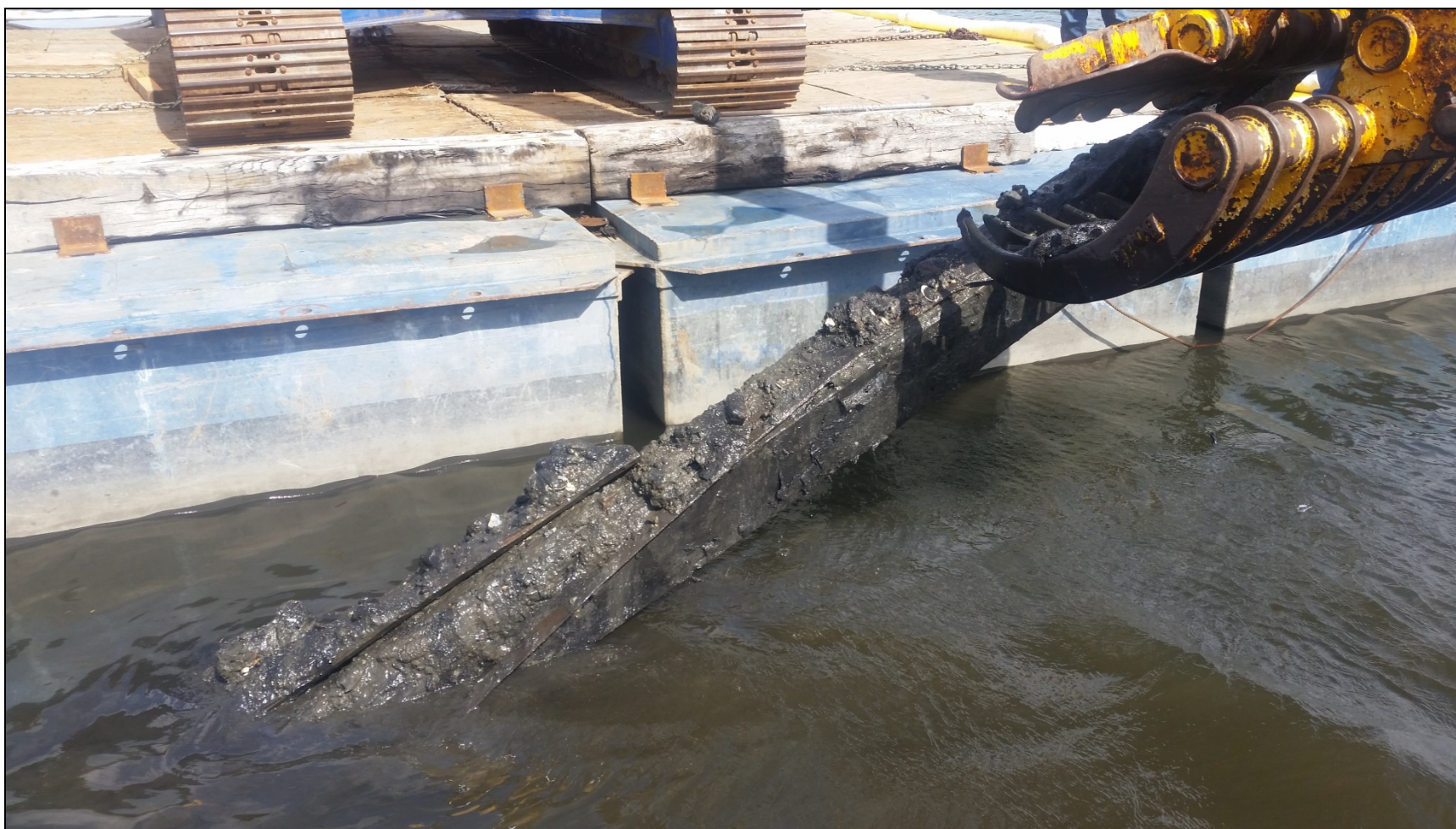
Figure . NBHSS Shipwreck #2 unanticipated discovery exposed during the debris removal phase of remediation activities within the of the 2015 Task 2 (Submarine Cable Crossing) Study Area of the NBHSS Upper Harbor (photograph by Joshua Cummings, Jacobs).
