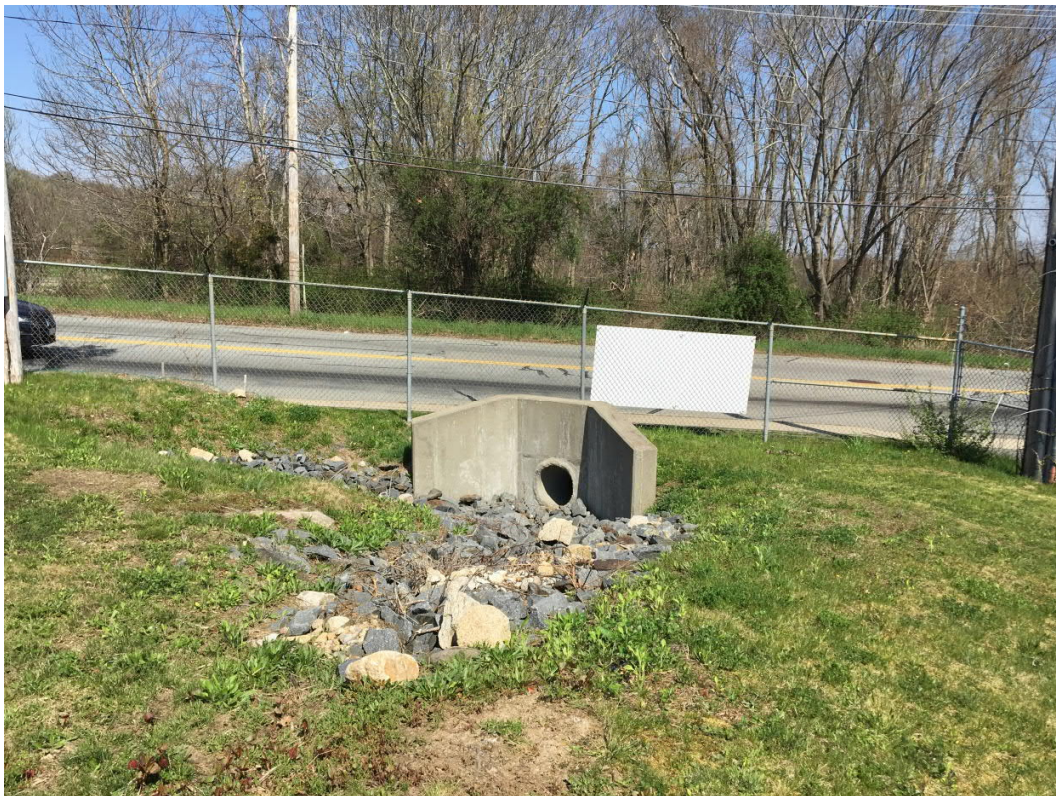
Culvert that receives run-on from portions of the western property boundary appears in good condition.
