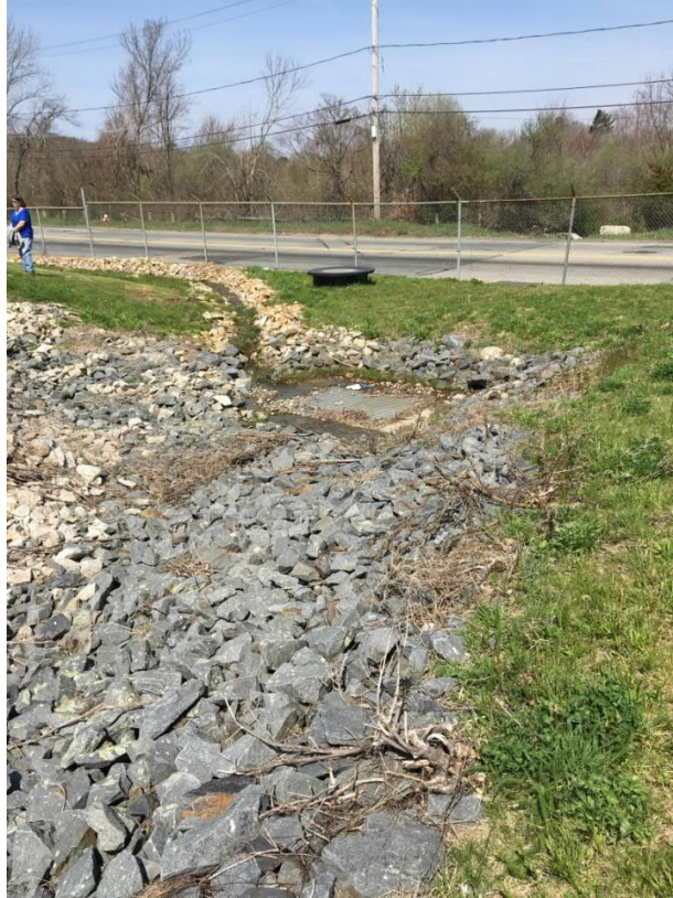
Inlet structure at Vault #2 which receives run-off from the cap collection swales.
