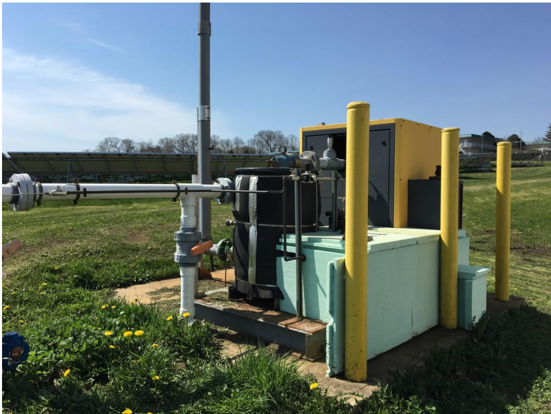
View of landfill gas extraction system blower and discharge stack
