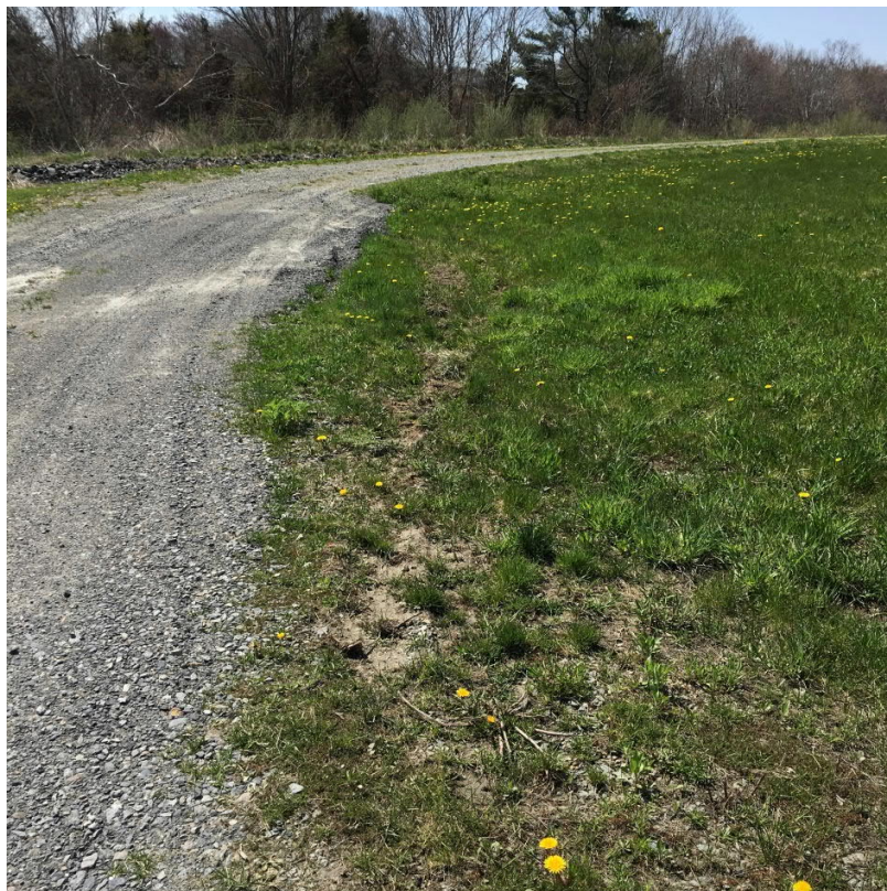
Minor rutting along edge of gravel access road in the southeastern area of the landfill cap should be filled and seeded.
