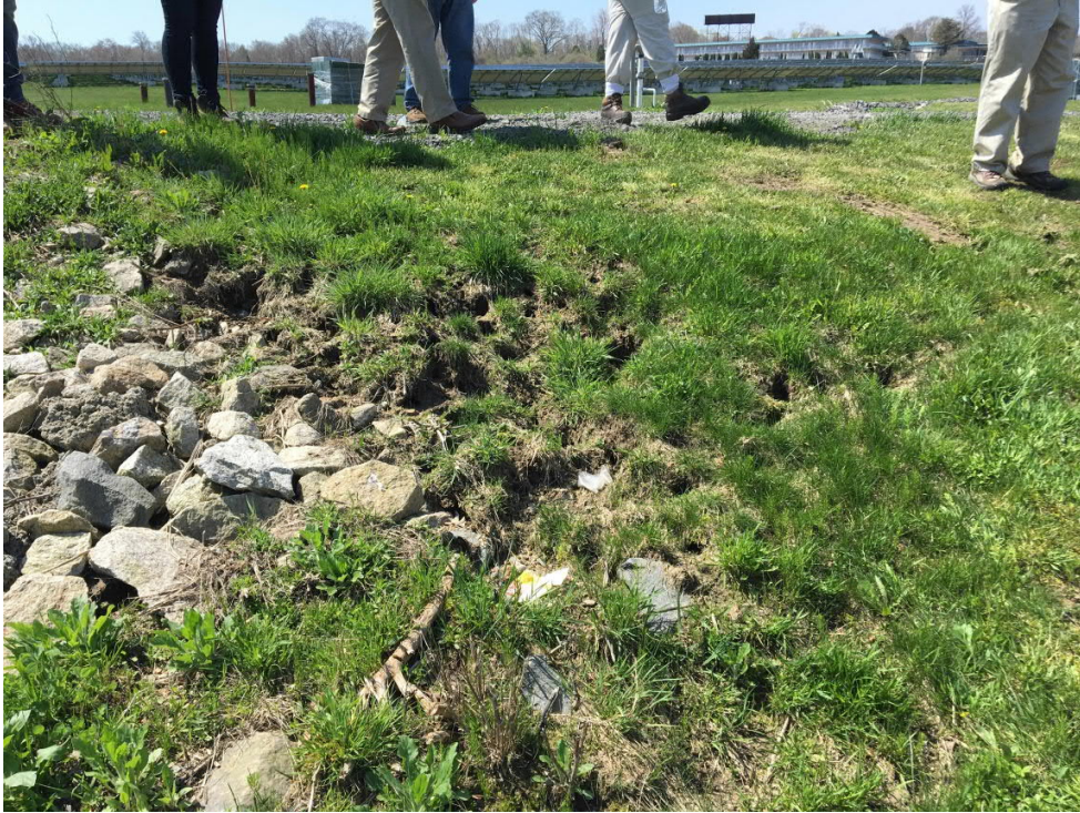
Small animal holes in cap adjacent to access road and inlet structure at Vault #2.
