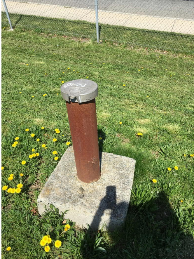
Piezometer PZ-10 not locked, but lock is present on concrete pad.
