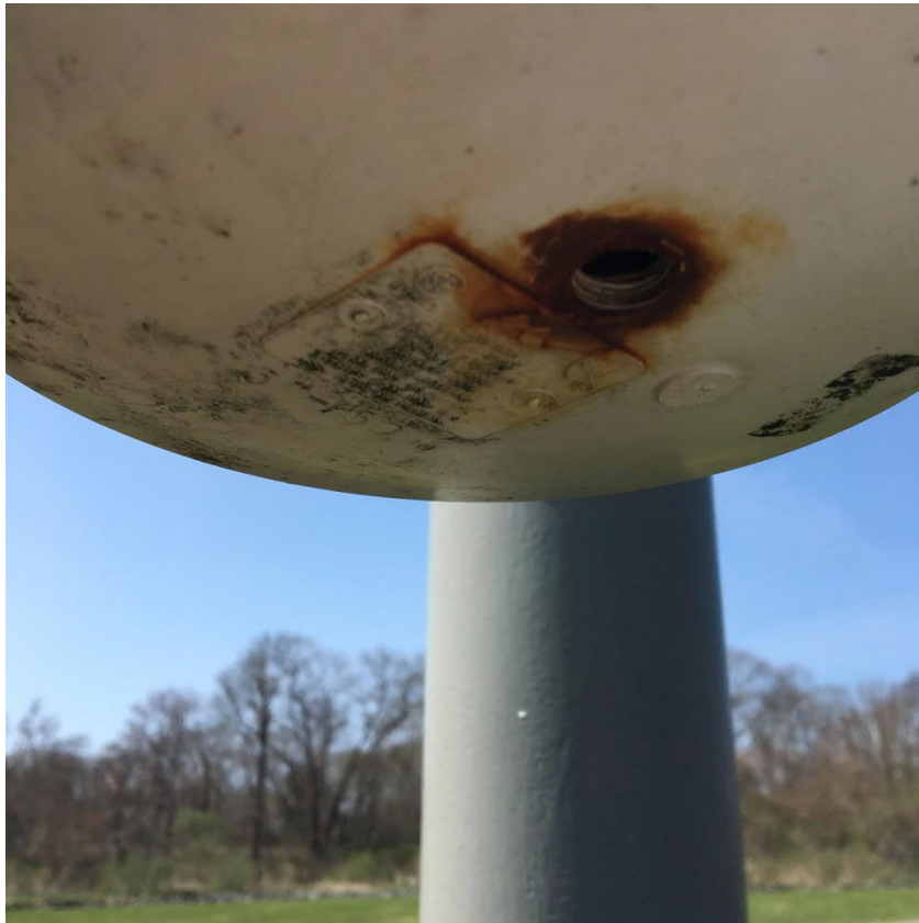
Cap on gas vent GV-11 is missing plug. Also, pipe coupling (not shown) connecting the vent pipe to the cap appears to have shifted, potentially impacting the seal.
