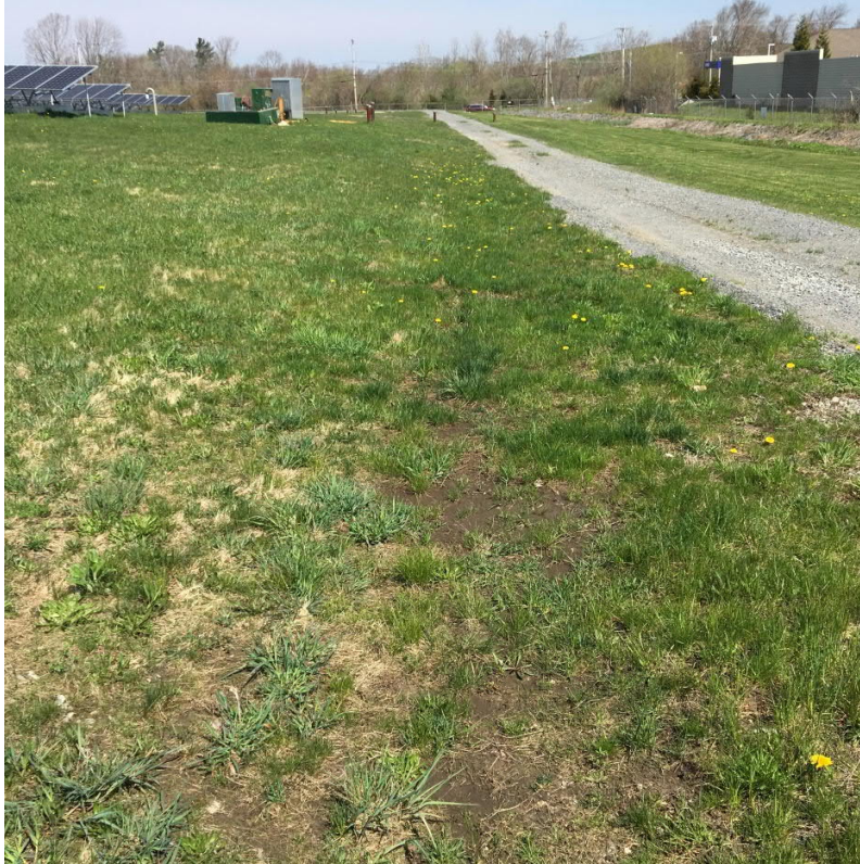
Small area of low vegetation and possible minor erosion adjacent to gravel access road in eastern portion of landfill cap should be filled and seeded.
