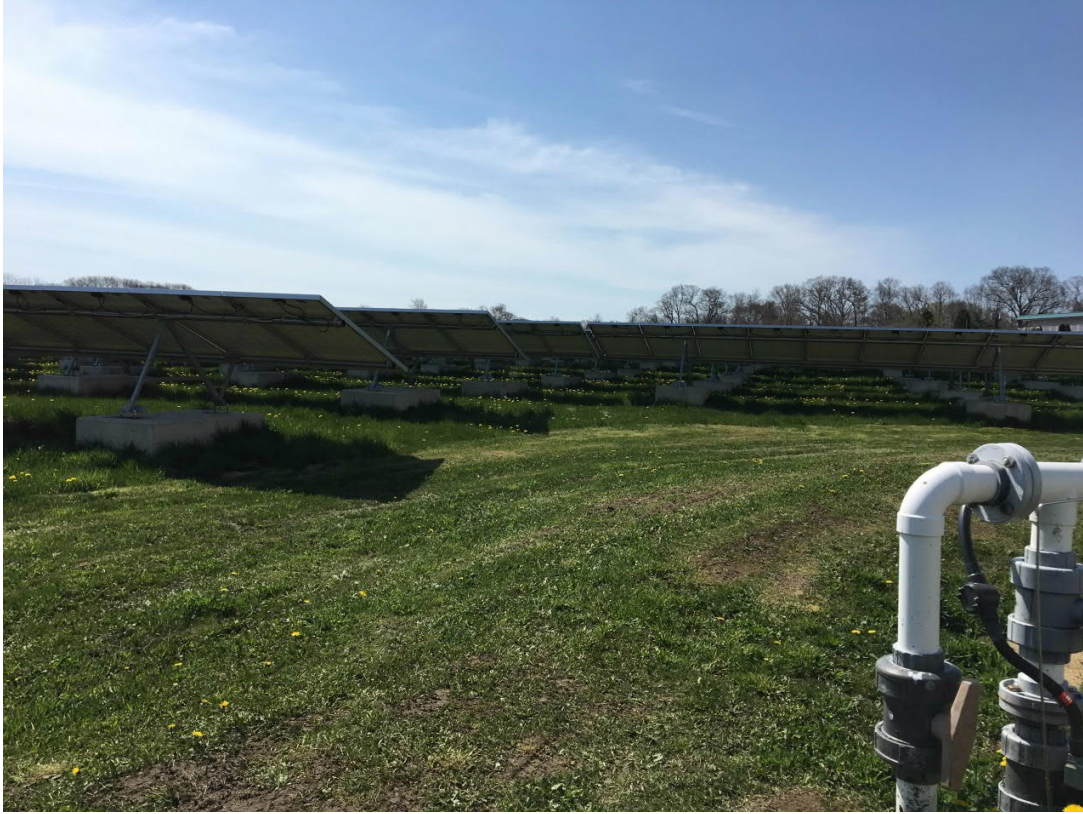
Minor areas of missing vegetation adjacent to landfill gas extraction system blower should be reseeded.
