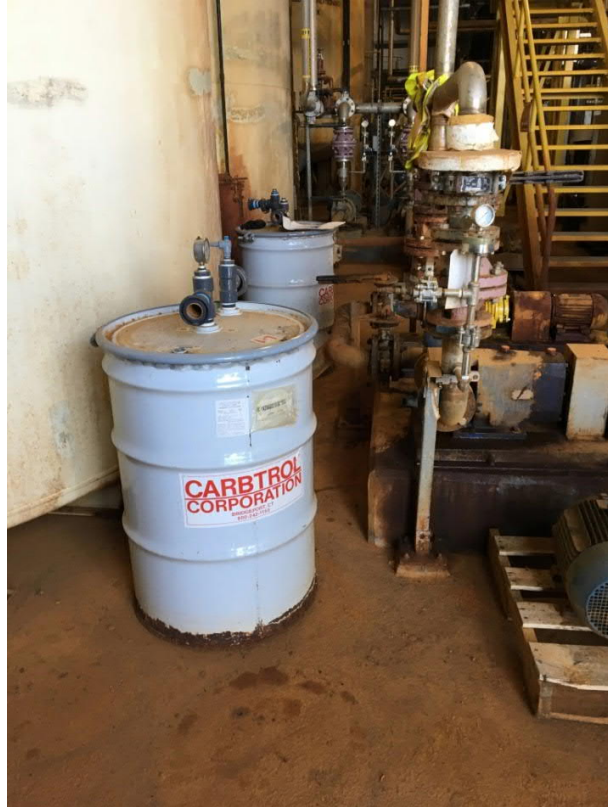
Spent granular activated carbon canisters from a former pilot test are rusting on the bottoms and should be removed from the GWTP for off-site disposal
