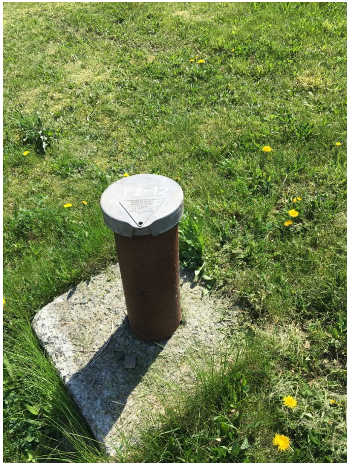
Piezometer PZ-12 not locked, but lock is present on concrete pad.
