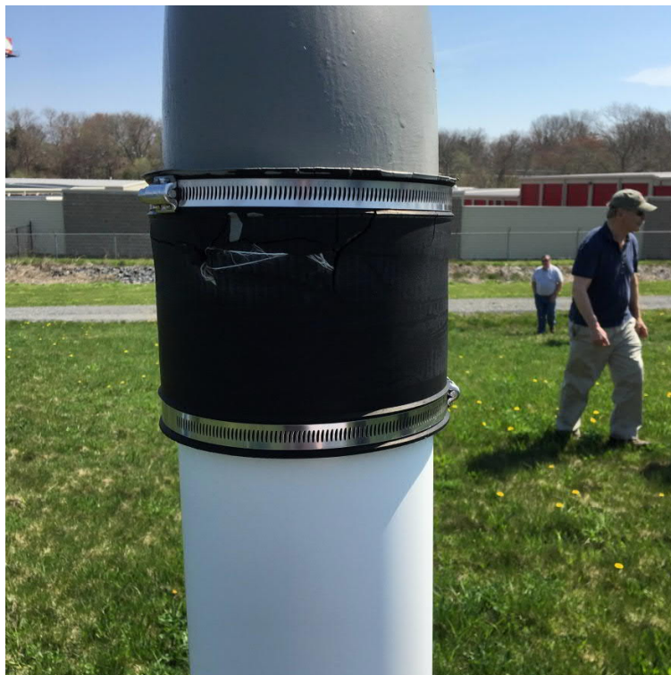
View of gas vent GV-3, which is directly connected to the gas extraction system header in the eastern portion of the landfill cap. Cracks in pipe coupling connecting the vent pipe to the extraction system piping resulting in an audible leak. The pipe coupling should be replaced.
