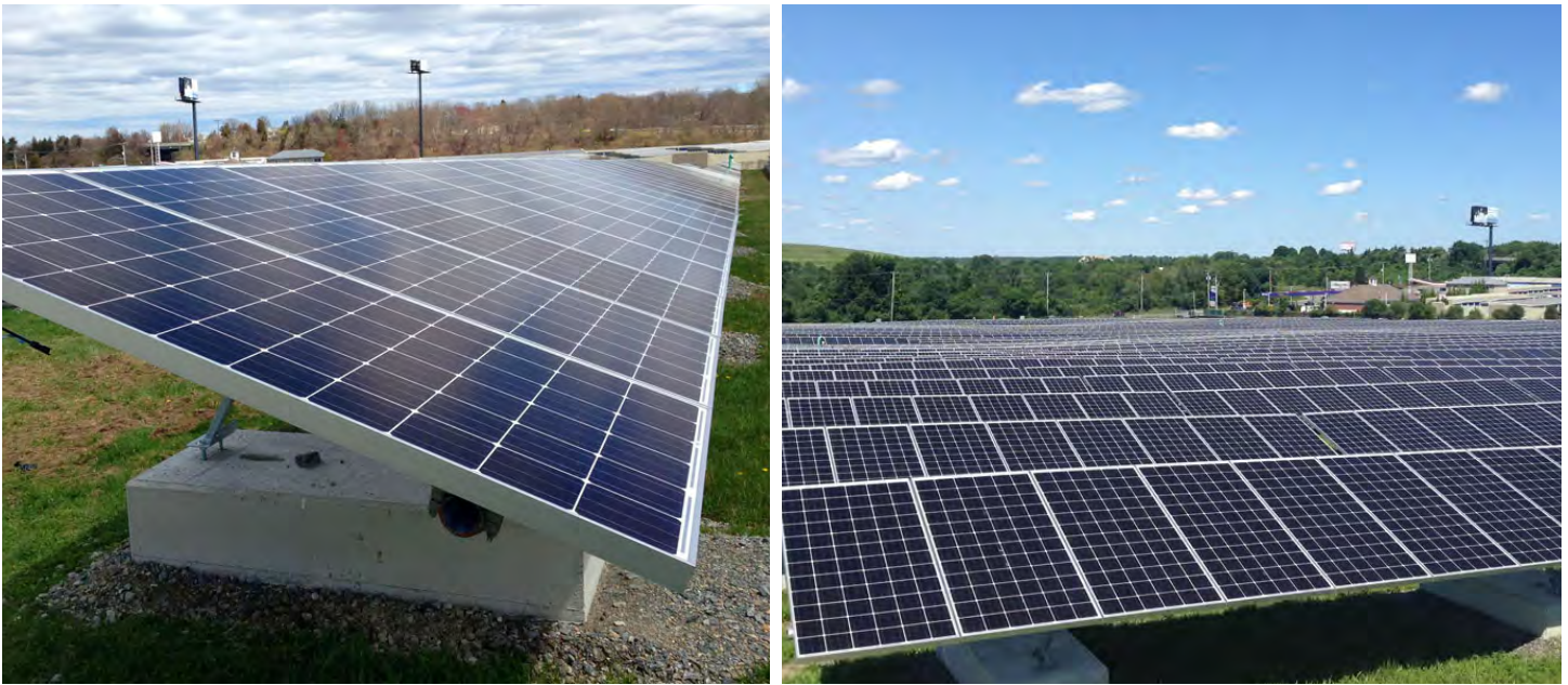
Figure 5. Over 5,000 block-mounted, fixed-tilt solar panels are in operation at the Sullivan’s Ledge site (Massachusetts).
