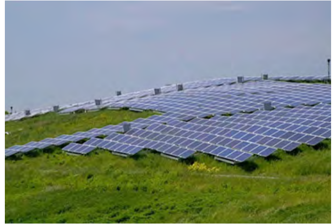
Figure 65. Solar array on Shaffer Landfill at the Iron Horse Park site (Massachusetts).
