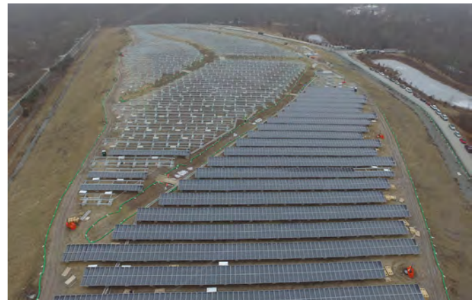
Figure 103. Aerial view of solar facility at the Rose Hill Regional Landfill site (Rhode Island). Photo used with permission of Kearsarge Energy.
