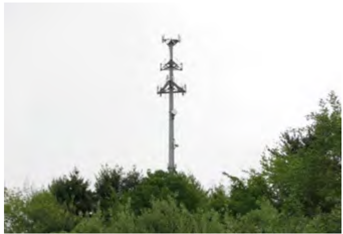
Figure 60. Cell phone tower on the CEC site (Massachusetts).
