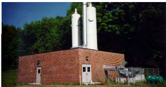
Figure 34. The groundwater treatment facility at the South Municipal Water Supply Well site.
