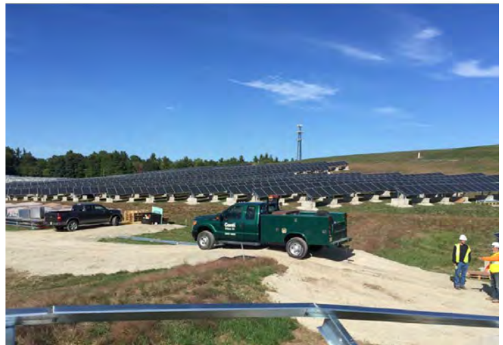
Figure 13. Installation of solar panels at the Charles-George Reclamation Trust Landfill site (Massachusetts).
